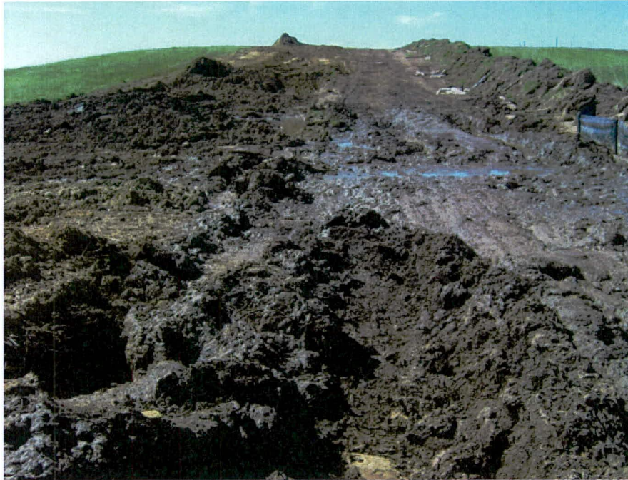
Photo 5 – Rutting Along the Right-of-Way
