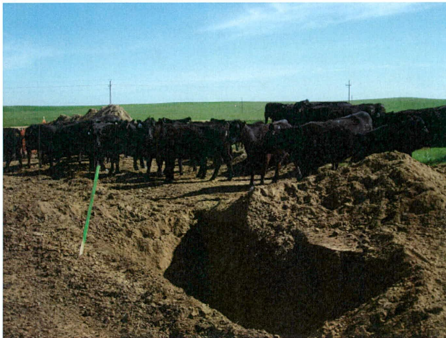
Photo 4 – Unsecured Trench near Livestock
