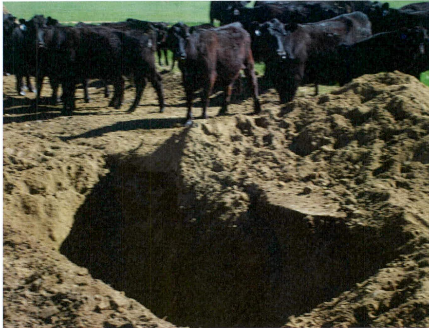
Photo 3 – Unsecured Trench near Livestock
