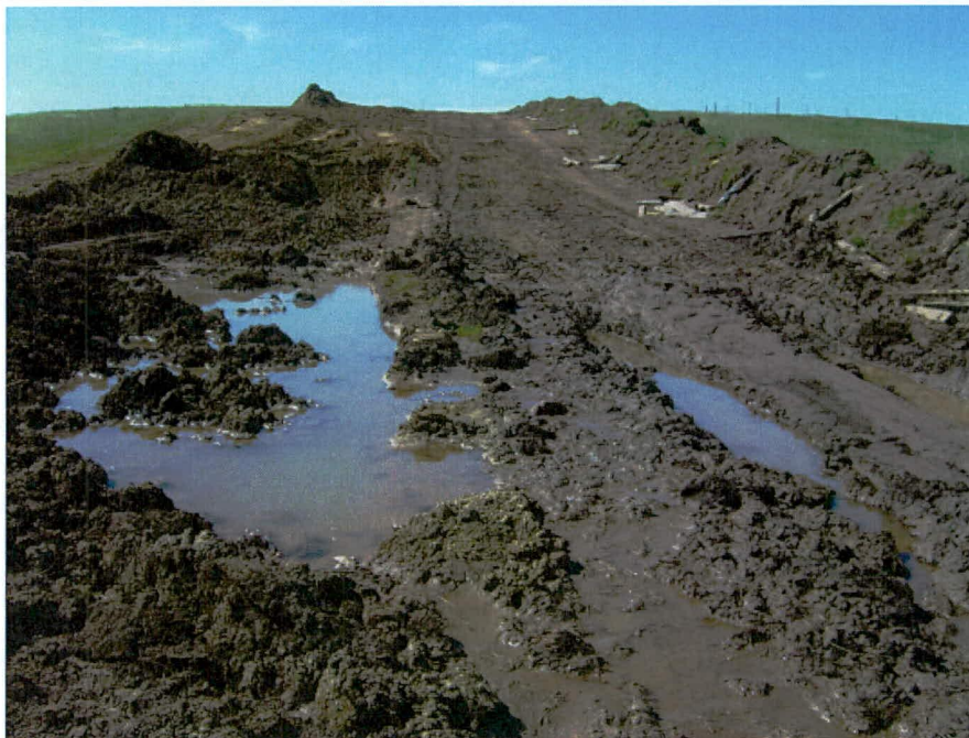
Photo 6 – Rutting Along the Right-of-Way
