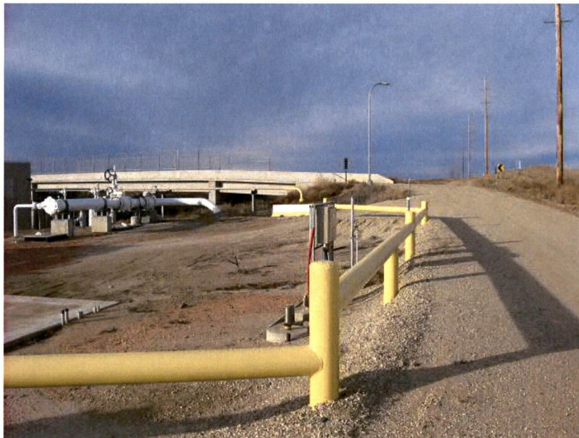
Photo 2 – Station 2016+34. View of interconnect facilities.
