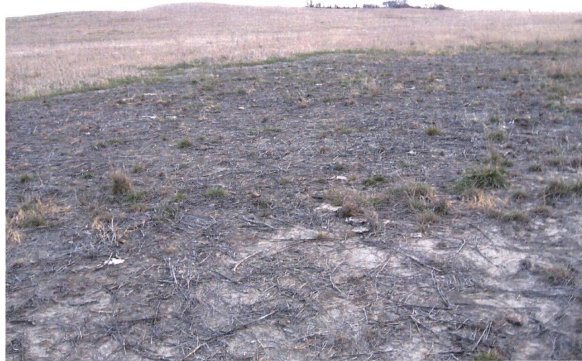
Photo 15 – Approx. Station 160+00. View of revegetation less than 70% south of 7 th Street SW.
