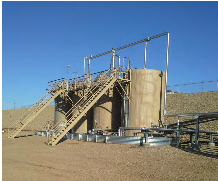
Photo 1. View of condensate storage area facing north.
