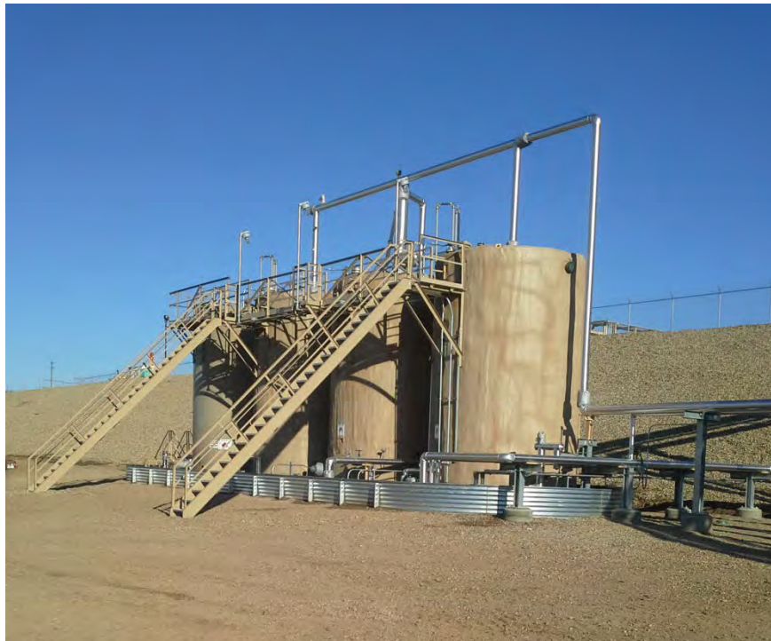
Photo 1. View of condensate storage area facing north.
