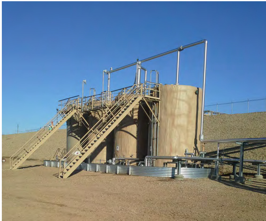
Photo 1. View of condensate storage area facing north.
