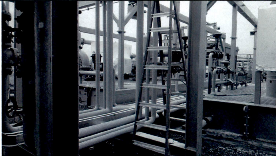
Photo 3: Distribution piping for new compressors
