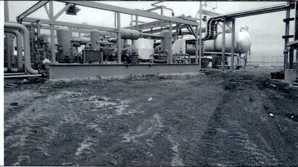
Photo 6: Disturbed soil in construction area.
