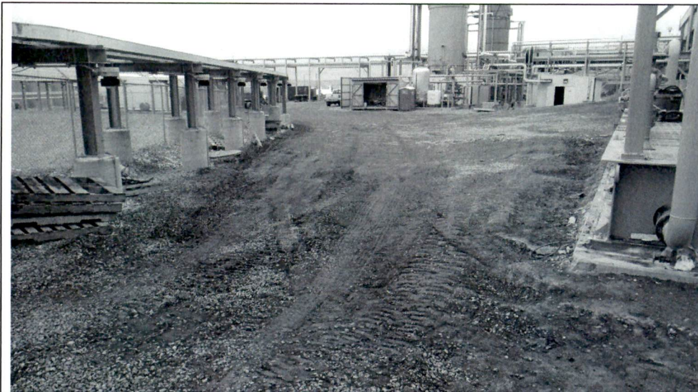
Photo 4: Disturbed soil in construction area.
