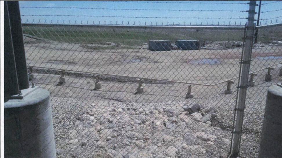
Photo 3: Rip rap drop that receives water from the area of the new compressors and discharges to the southeast.
