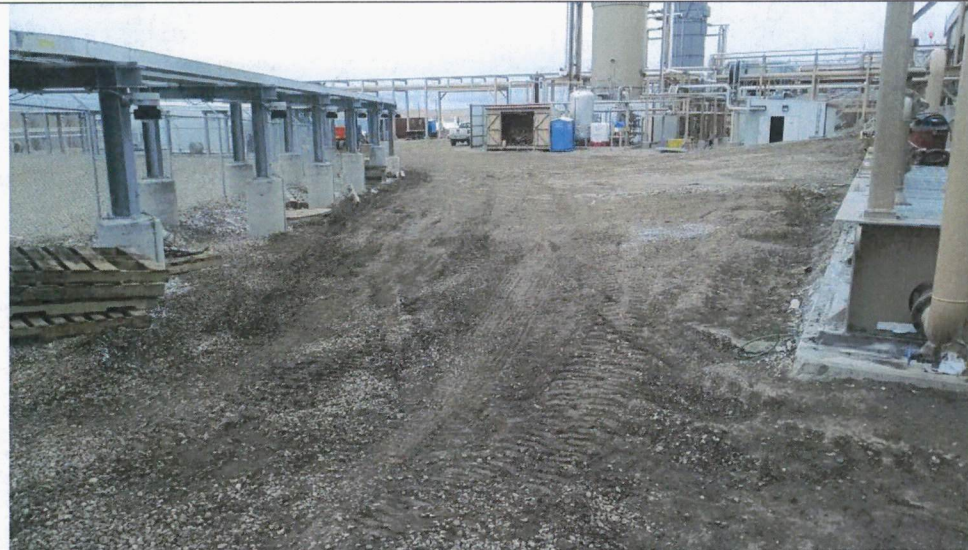
Photo 4: Disturbed soil in construction area.
