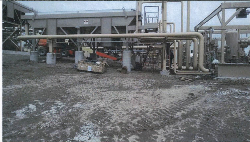
Photo 5: Disturbed soil in construction area.
