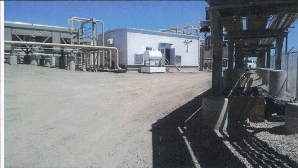
Photo 2: New compressor building and lube oil tank
