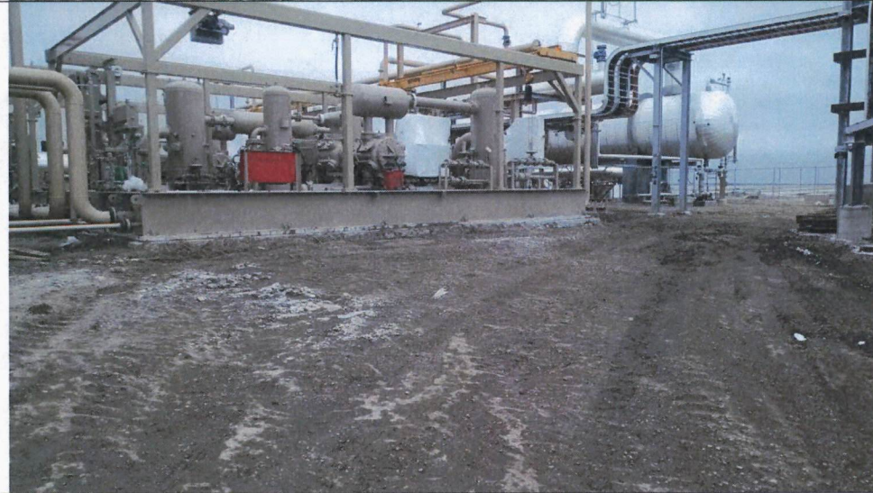
Photo 6: Disturbed soil in construction area.
