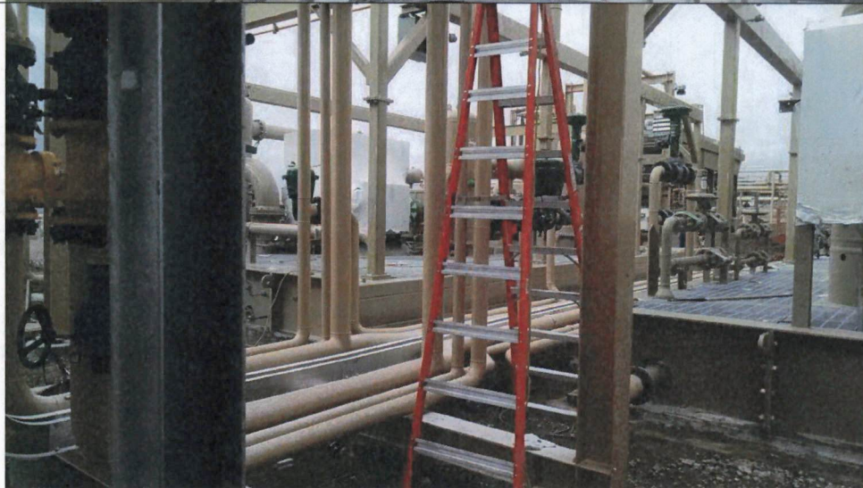
Photo 3: Distribution piping for new compressors
