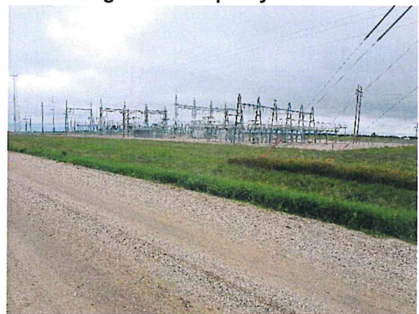
Existing MDU Substation Photo 12 Looking NE
