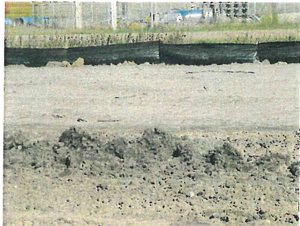
Photo 14 East Prop. Line Erosion Control at Road ROW
