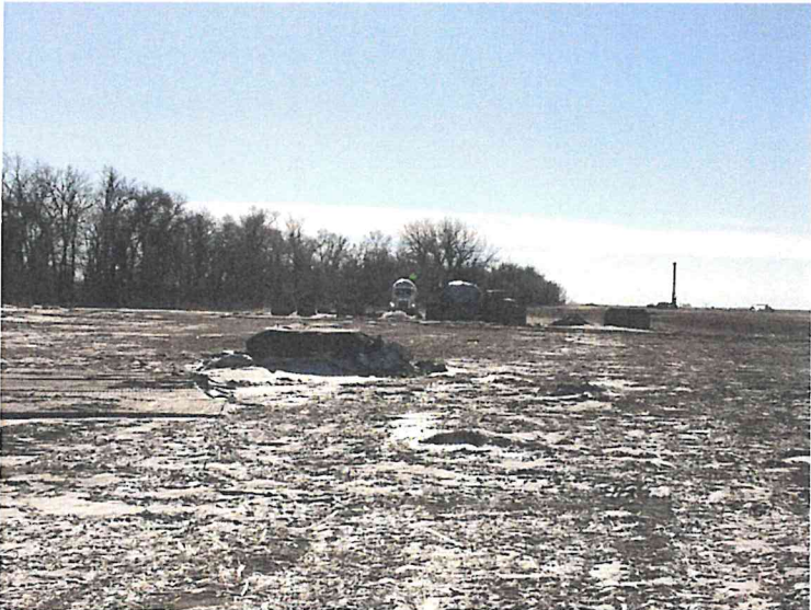
Thermal blankets placed over the foundation to prevent freezing. Foundation No. 7 Looking S.
