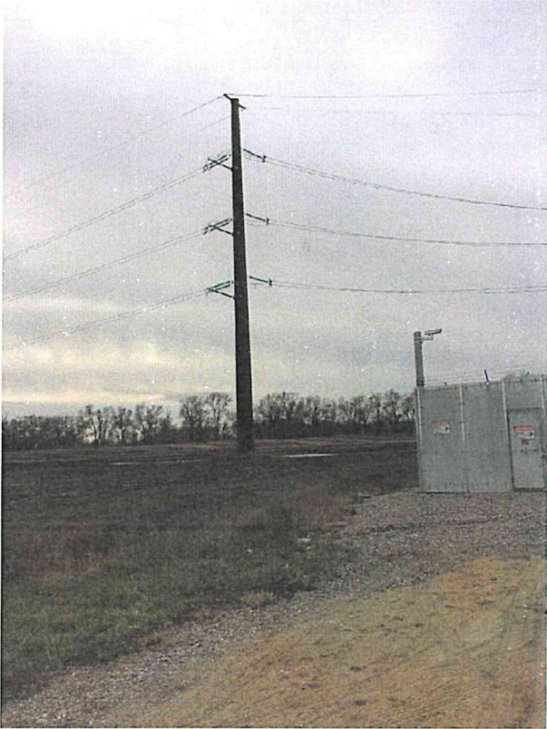
Power Pole No. 001 Looking W.
