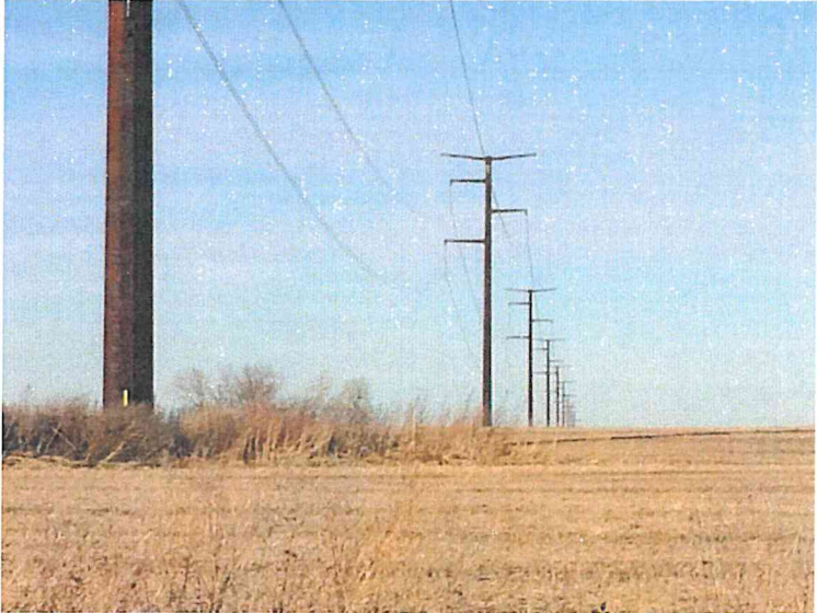
Power Pole 041, 040, 039, 038, 037, 036 Looking N.
