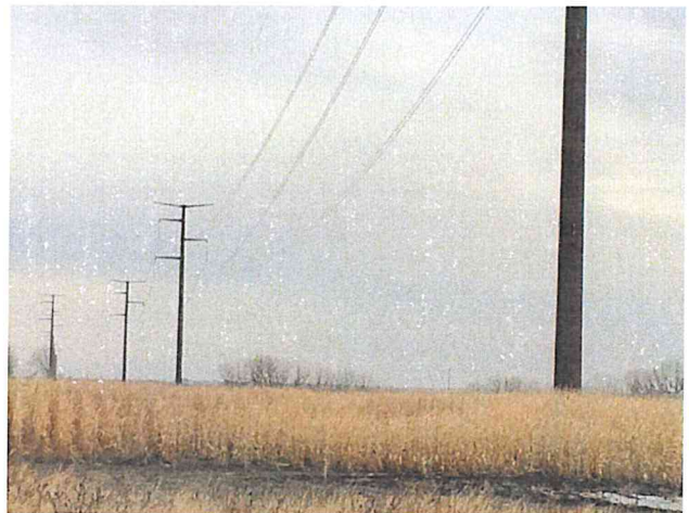
Power Poles 020, 021, 022, 023 Hwy 281 Looking E.
