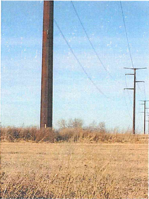
Power Poles Base 041 Looking North
