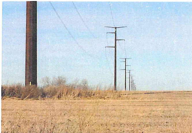
Power Poles 037, 038, 039, 040, 041, 042, 043 Looking N.
