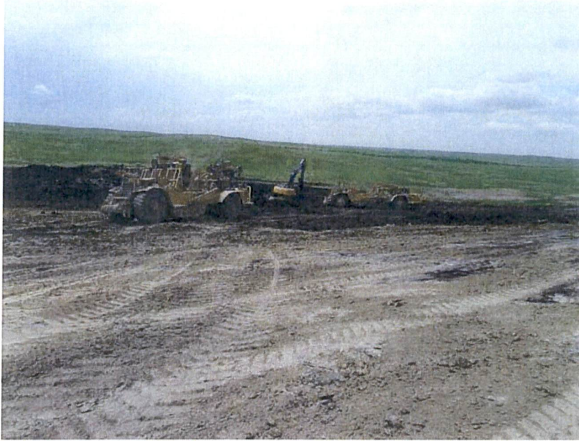
Photo 1: This cut is for a new haul road. Topsoil and subsoil are being removed from the sides as the existing haul road is widened to connect to Permit BNCR-1101 at the Center Mine. Topsoil is being removed and separated. Dozers separate topsoil using color as a guide. The backhoe loads soil into scrapers for direct respreads in the “Butterfly Pit”. Approximately 60 inches of topsoil and subsoil are being removed.
