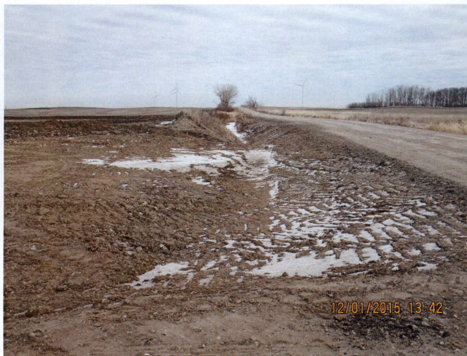
Figure 6. Photo of a ditch to be regraded to establish better runoff collection near T27.
