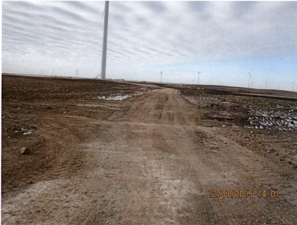
Figure 9. Photo of the gradual cut in the service road to promote better drainage and still allow safe access to the turbine.
