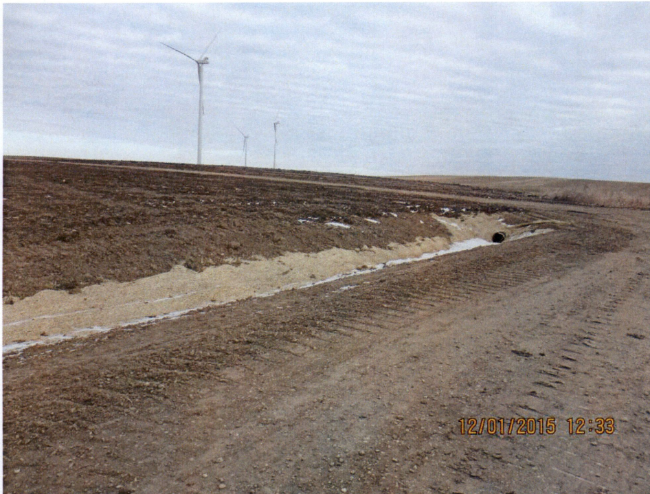
Figure 1. Photo taken of reclaimed service road radii corner. Drainage ditch has been graded, erosion mat in place, and culvert installed.
