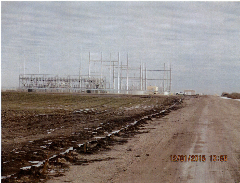
Figure 8. Photo of completed substation and work still needed to reclaim the service road and topsoil around it.
