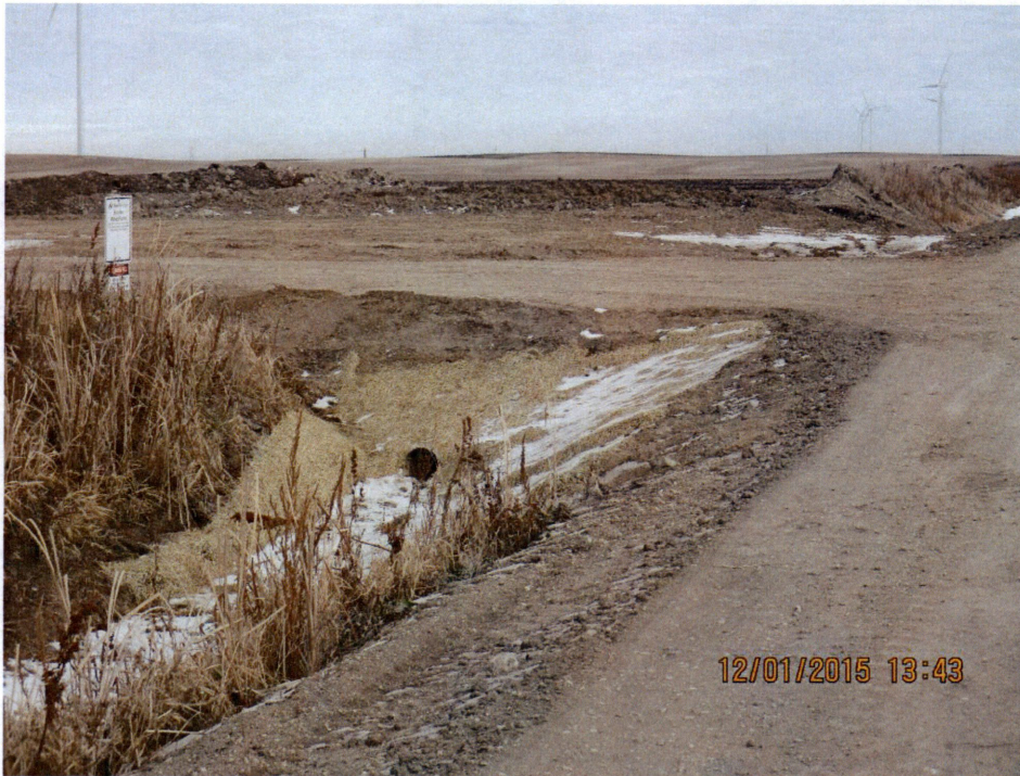
Figure 7. Other side of the service road of T27 with culvert and erosion mat in place.
