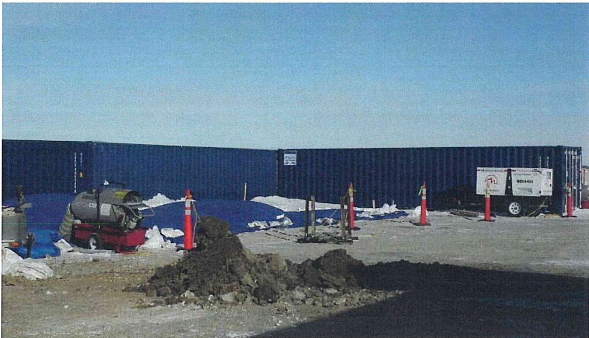
Substation Ground Heating
