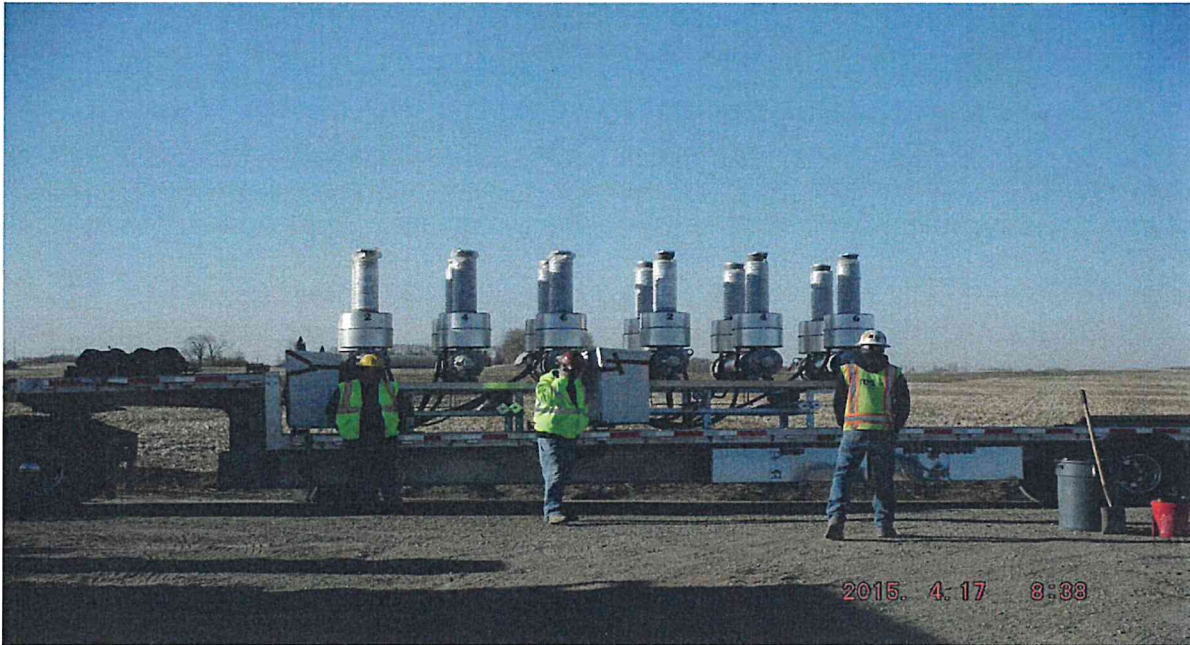
Substation – Low voltage breaker delivery
