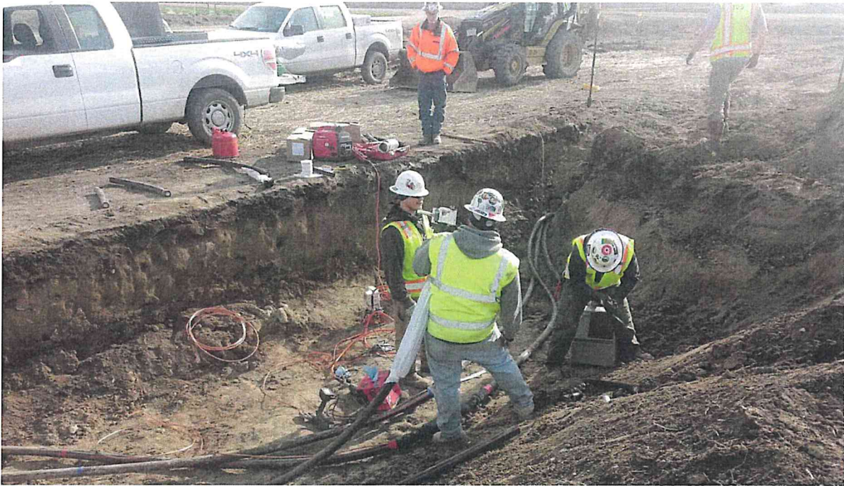
Collection System – Circuit 5 splice termination
