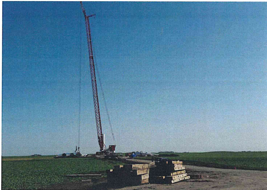
Main Crane - T25
