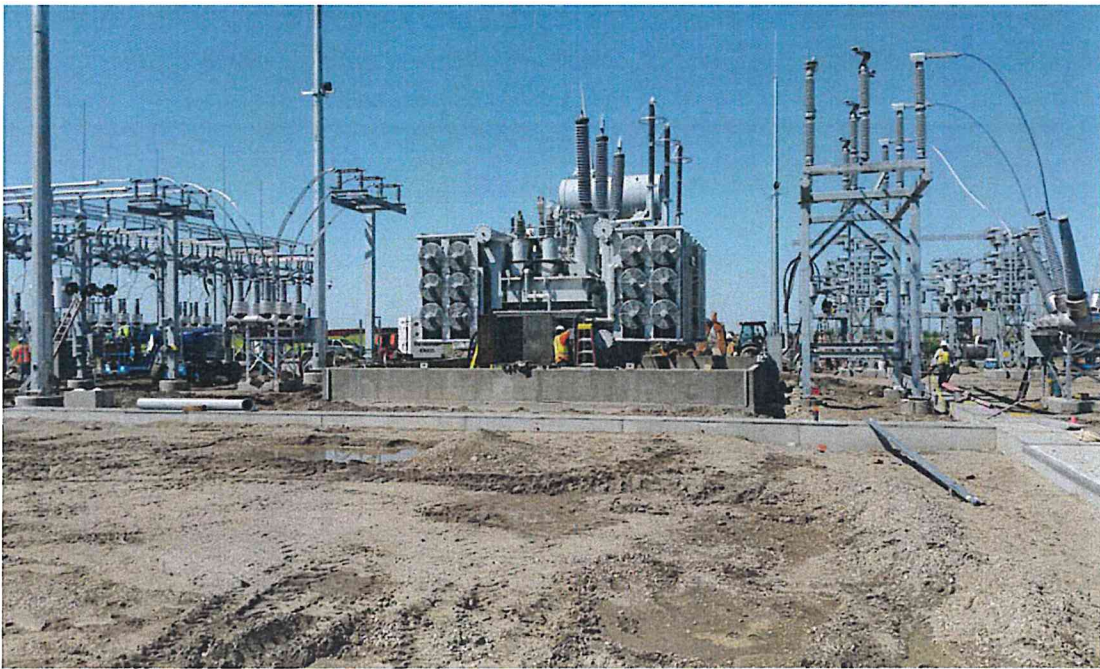
Substation – Transformer Testing
