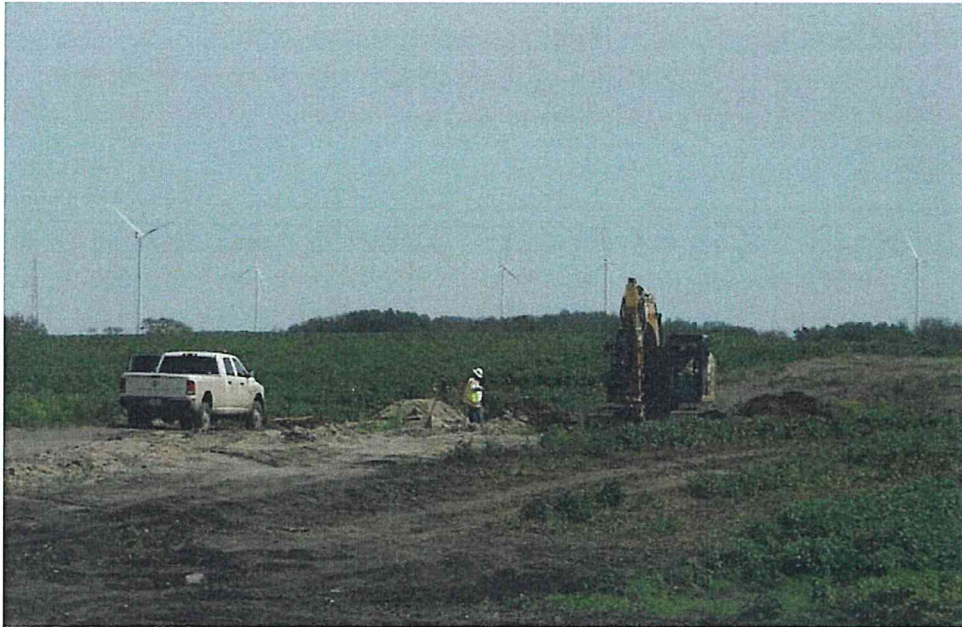
Cable splice between T13 and T12
