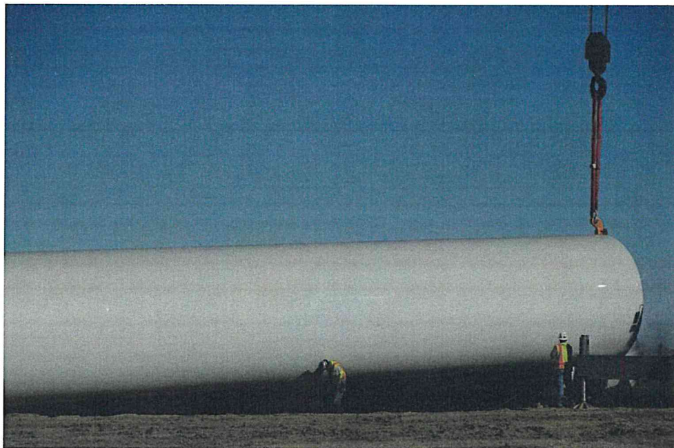
Cleaning Tower Section at T61
