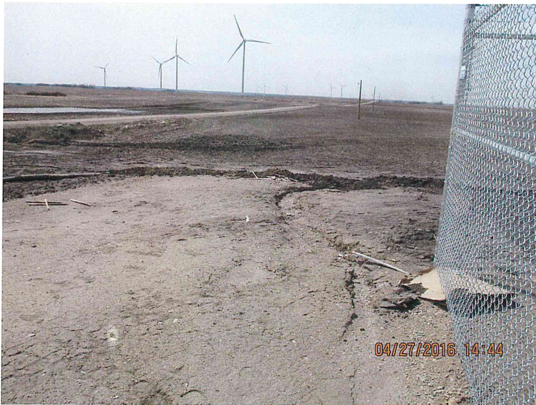
Figure 13. A more permanent channel will be installed to prevent further washouts at this southwest corner of the O&M building.
