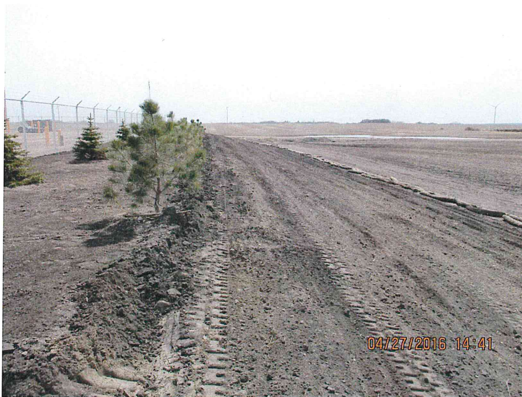
Figure 11. Trees around O&M building planted. Straw swaddles will be moved to the top of the slope once ECB is in place.
