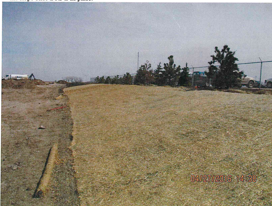
Figure 12. ECB anchored and stapled in place on the slopes surrounding the O&M building.
