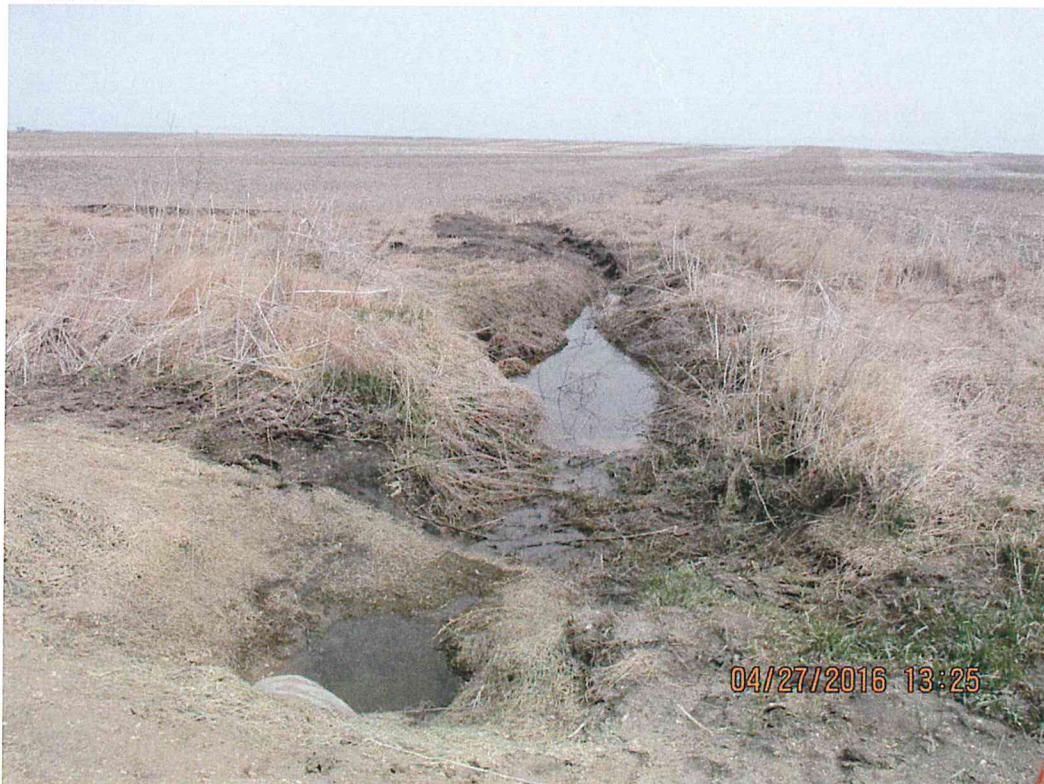
Figure 8. Small trench dug to alleviate water backup at culvert on 53 rd Ave NE near T48 and 49.
