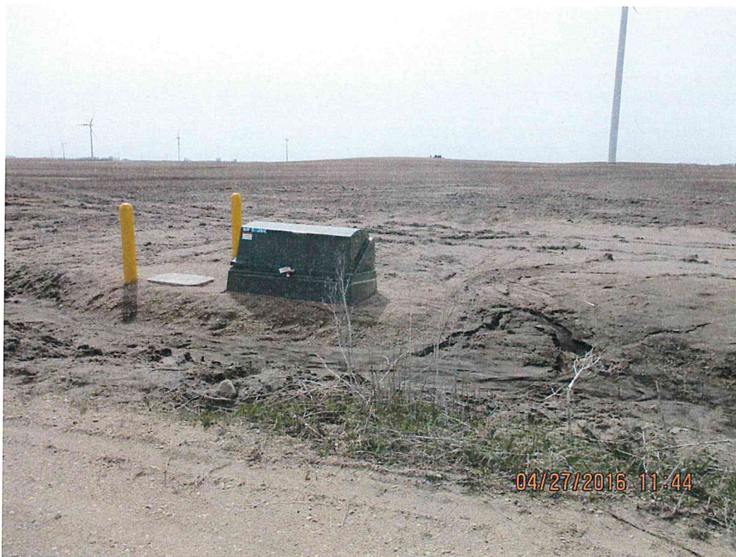
Figure 1. Photo of area surrounding a junction box that needs some maintenance due to runoff and settling.
