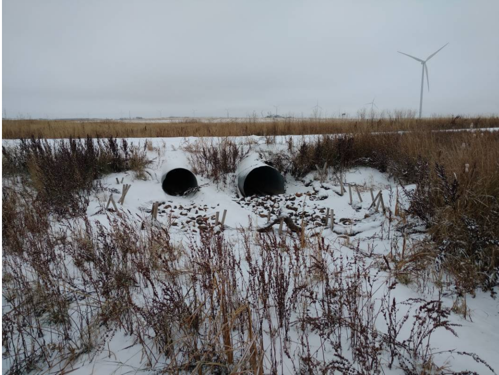
Figure 12. Photo taken facing west at 53 rd Ave. The road at this location was identified in the May Construction Inspection report (Figure 14) as being impacted by construction traffic. Road has been restored and riprap was placed at culverts.
