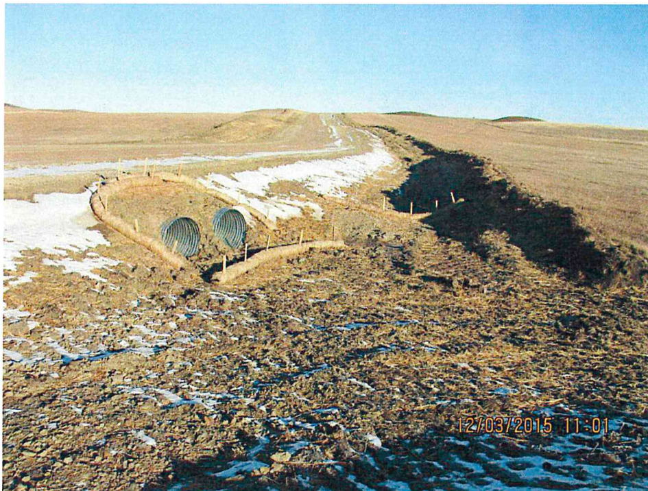
Figure 2. Two new culverts installed on service road between T3 and T4. ECDs properly installed to prevent erosion problems.
