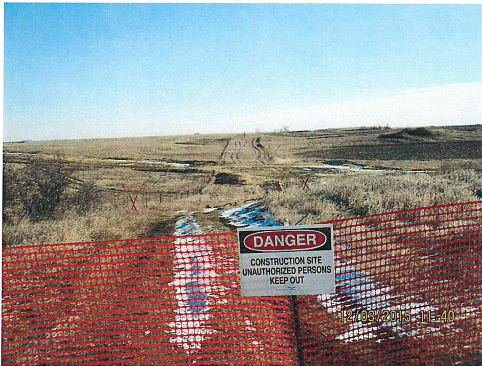
Figure 9. End of construction work area for the winter. ECDs and safety barrier in place.
