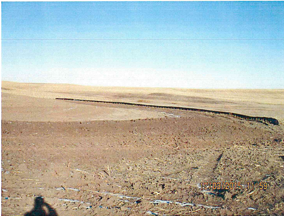
Figure 11. ECDs installed at the edge of working area preventing sediment from leaving the working area.
