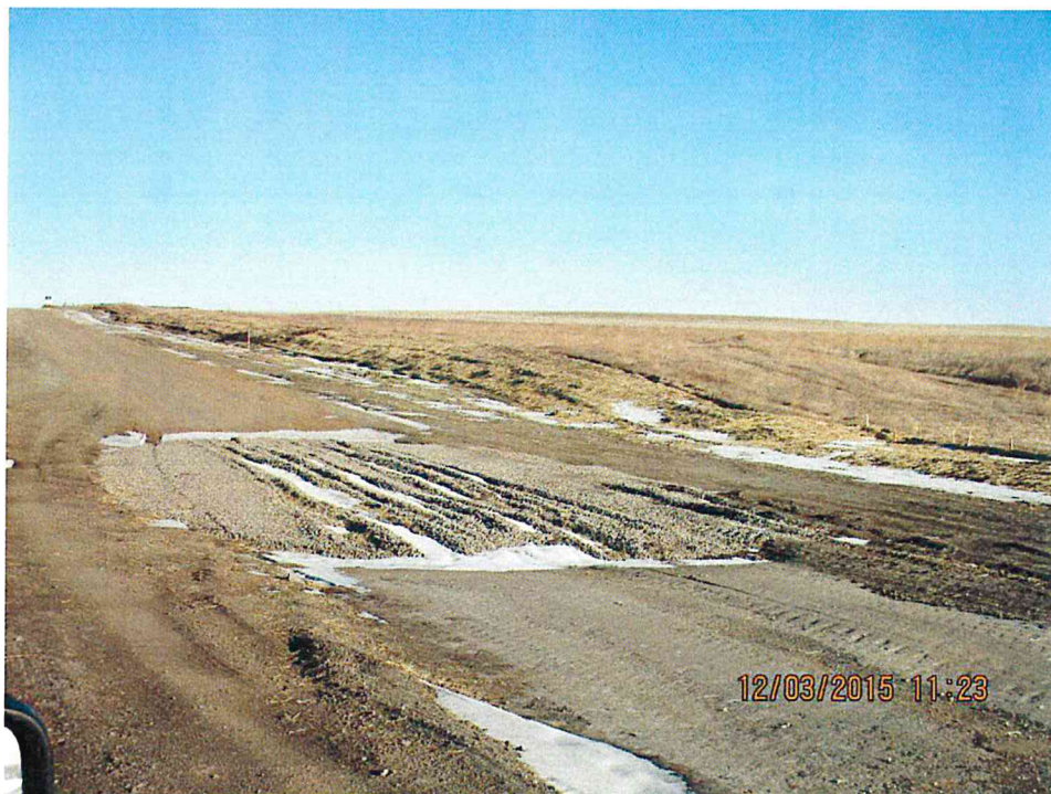
Figure 6. French drain installed in the service road perpendicular to the drainage path crossing the project area.
