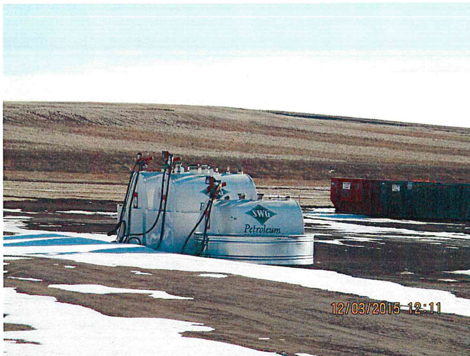
Figure 12. Fuel tanks in containment at laydown yard.
