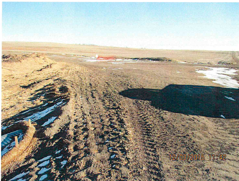
Figure 10. Access road radii increased to accommodate turbine deliveries for turbines T17-T20. These will be regraded and reclaimed at the end of construction.
