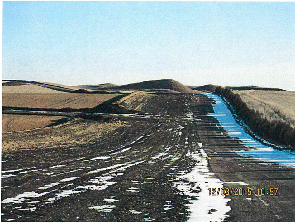
Figure 1. Photo of cleared topsoil along service road ROW. Mulch anchored in for erosion protection.
