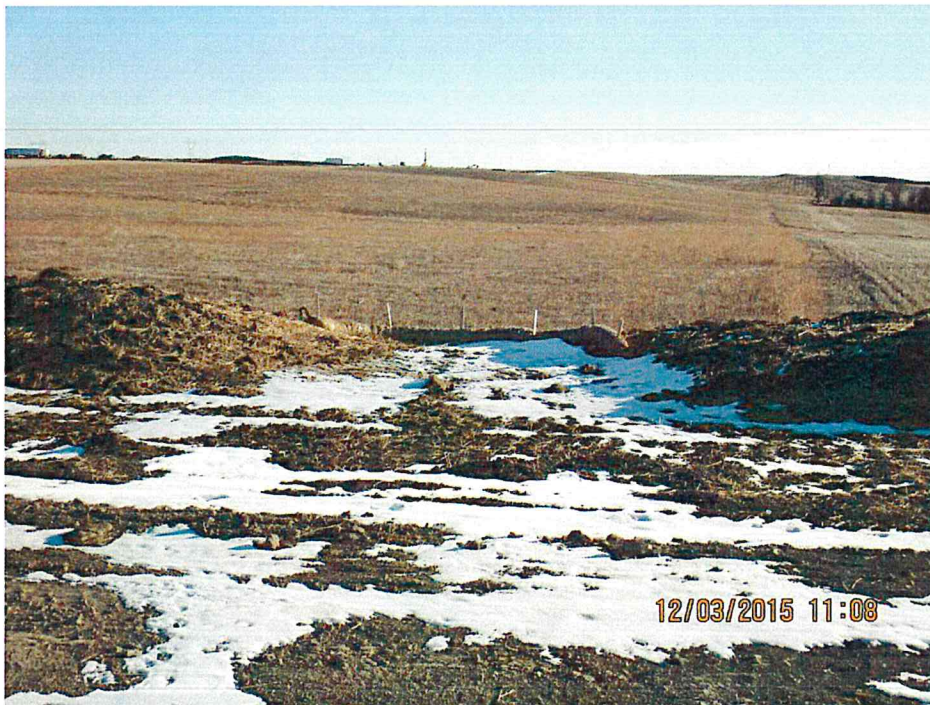
Figure 3. Break in the topsoil berm to alleviate storm water runoff. Straw swaddle in place to prevent sediments from exiting working area.
