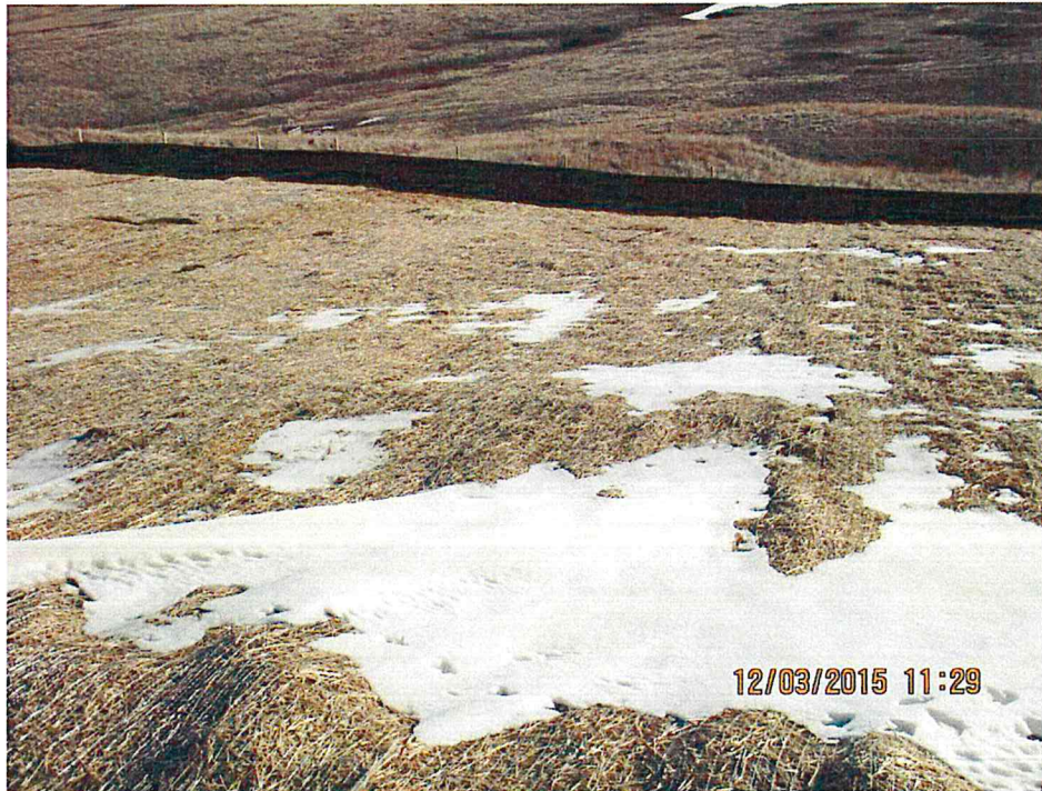
Figure 7. ECDs installed on back slope of T20.
