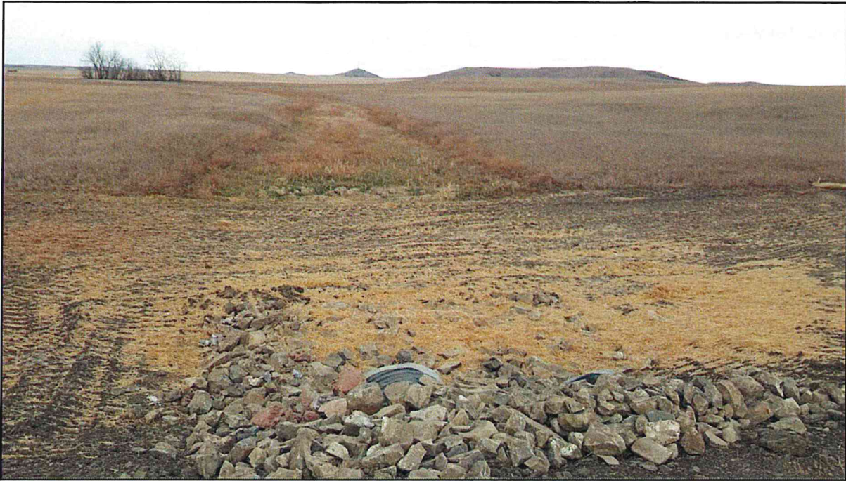
Figure 3. Rip-rap that was installed up-drain of the culvert found between T2 and T3.
