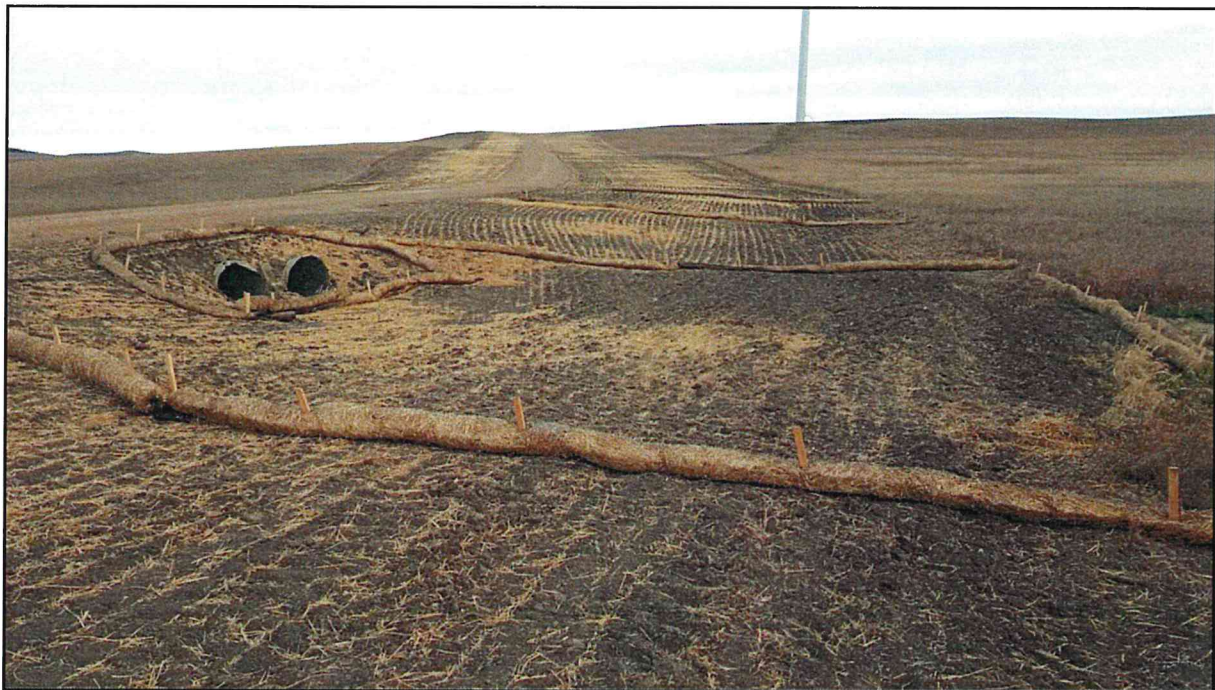
Figure 2. Culverts found between T3 and T4. ECDs were properly installed to prevent erosion.
