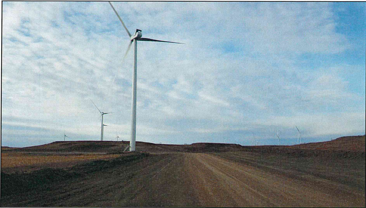
Figure 5. All 52 turbines have been completed and put in place. Only 4 of the 52 turbines are yet to be mechanically completed.
