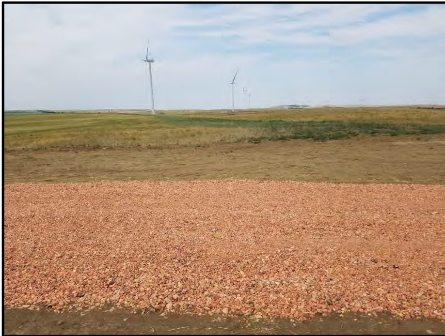
Photograph 8. View looking west along an underground collection line in the southwest 1/4 of Section 21, T139N, R39W.
