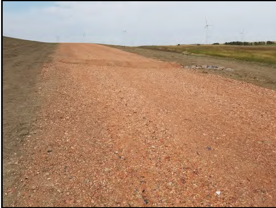
Photograph 5. View of water diversion erosion control device placed in the access road along with a French drain.
