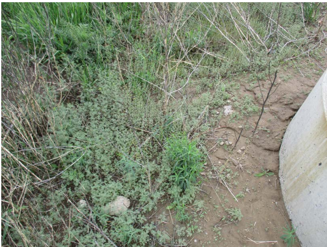
Below: Photo 12 (Structure 1391D Point 431) – Observe small chunks of concrete waste and small flow paths forming around structure base.
