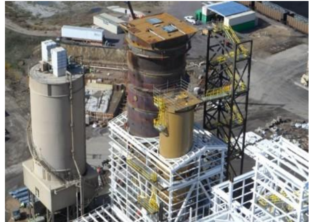
10-07 Waste ash/pebble lime silos
