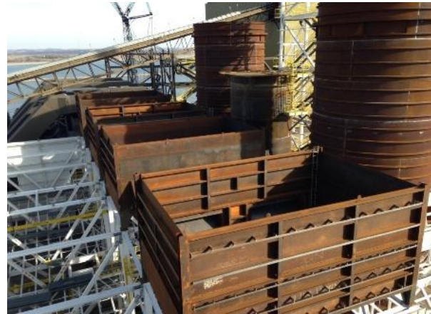
11-04 Lower baghouse modules, hydrated lime silo & scrubber
