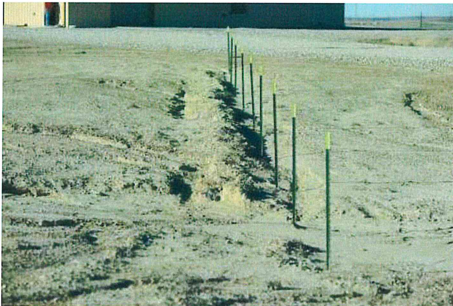
Photo 2: Facing north entrance to facility, erosion from parking lot runoff.
