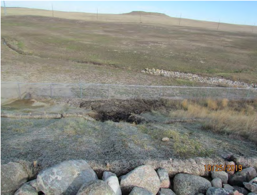
Photo 27: Slope failure. Top of hill view of photos 1-3
