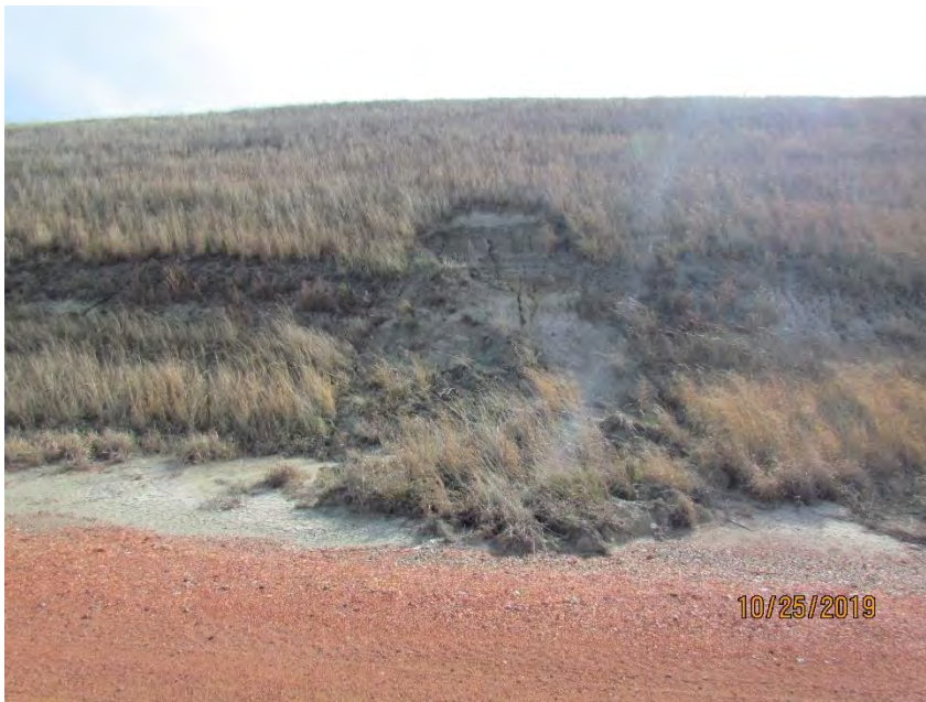
Photo 34: Slope failure along the southcentral extents of the facility boundary
