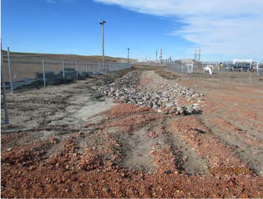
Photo 45: Stormwater impacts near the facility's eastern fence line
