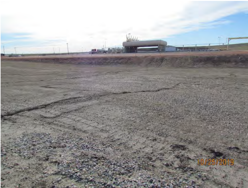
Photo 14: View of surface water drainage gully formation
