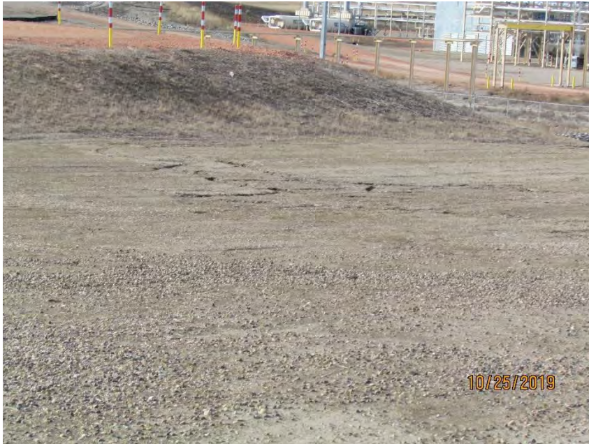
Photo 13: View of surface water drainage gully formation
