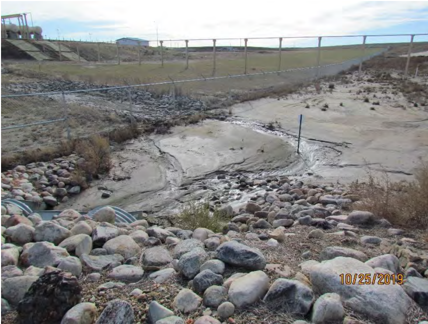
Photo 19: Stormwater flow paths and Sediment draining to culvert within eastern portion of facility site 10-25-2019
