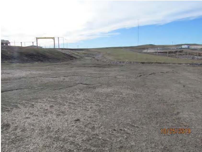
Photo 15: View of surface water drainage gully formation
