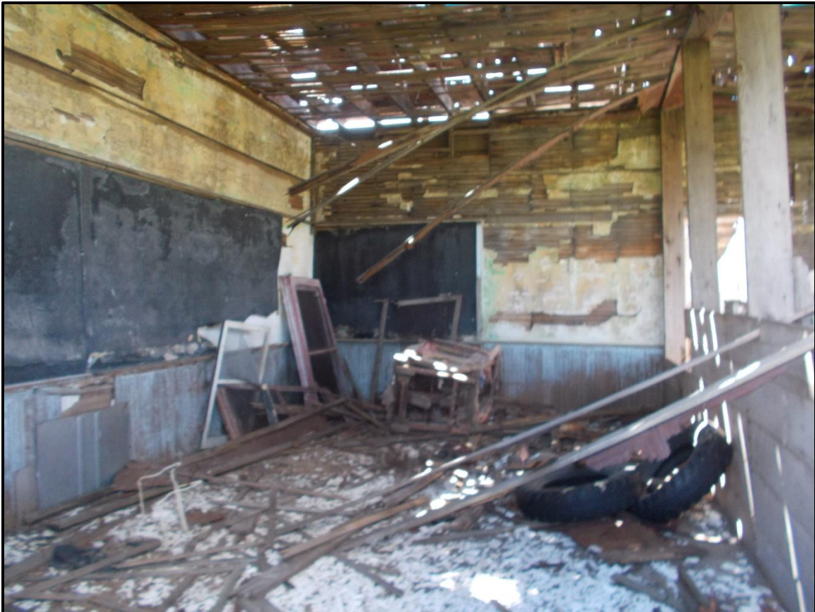
Figure 21: Interior of the former schoolhouse. Note chalkboards, deteriorating lathe and plaster, and wood-frame partition which are likely to have been constructed at a later date.
