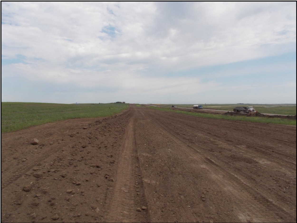
Figure 9: Overview of the Summit Midstream Energy Divide Lateral pipeline corridor in Section 11, T. 161 N., R. 100 W., Divide County. View is to the north. The pipeline is in place at this location and remediation activities were in progress at the time of survey.
