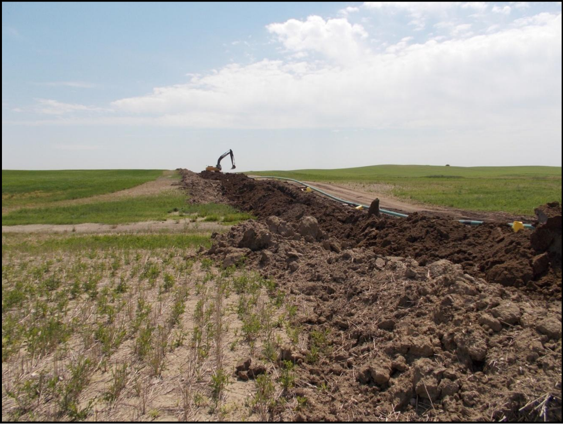
Figure 10: Overview of construction activity within the project corridor and adjacent agricultural fields. Photograph taken in Section 9, T. 160 N., R. 100 W., view to the south.
