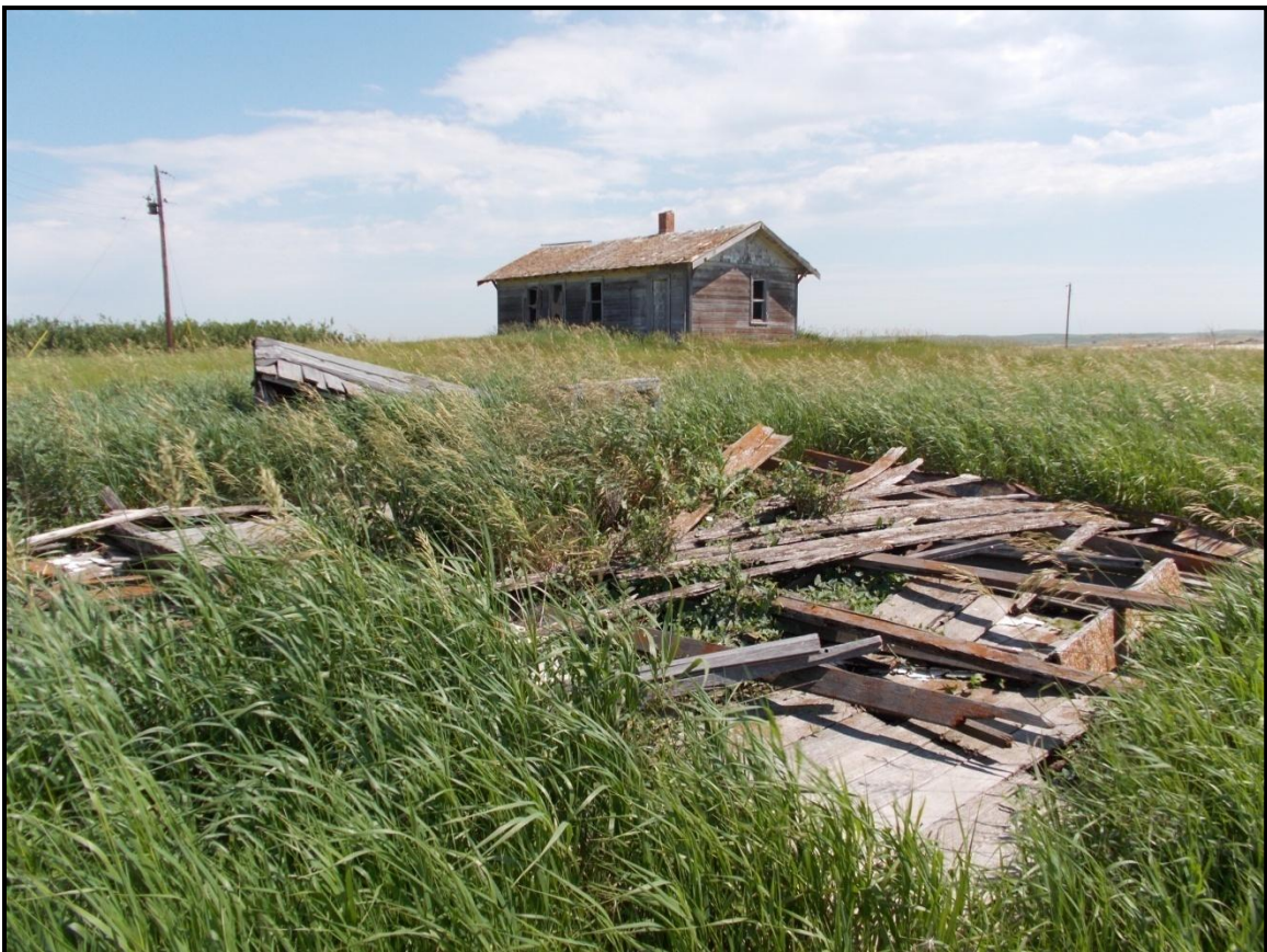
Figure 17: Overview of collapsed wooden structure at 32DV129 with farmhouse in background, view to the northeast.
