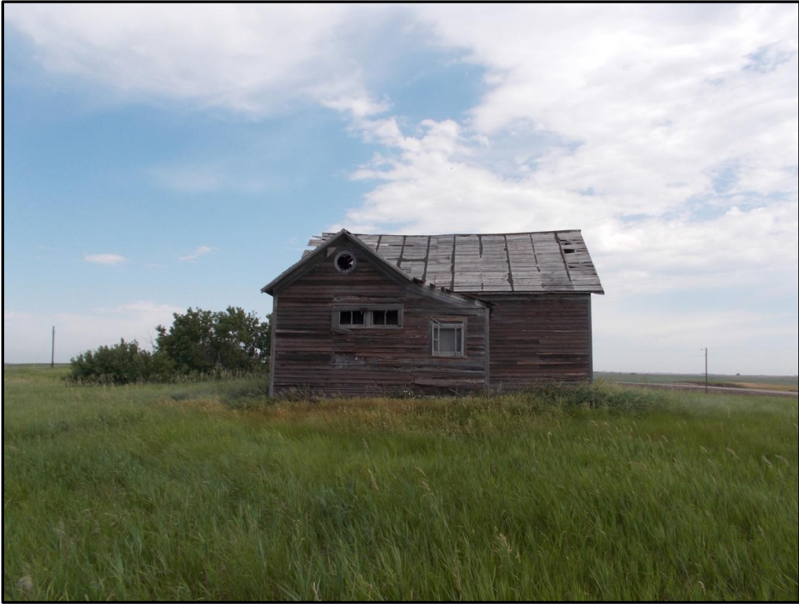
Figure 20: Overview of the schoolhouse which displays that the entrance has been infilled and a shed (lean-to) foyer added to accommodate the new, east-facing door is visible.
