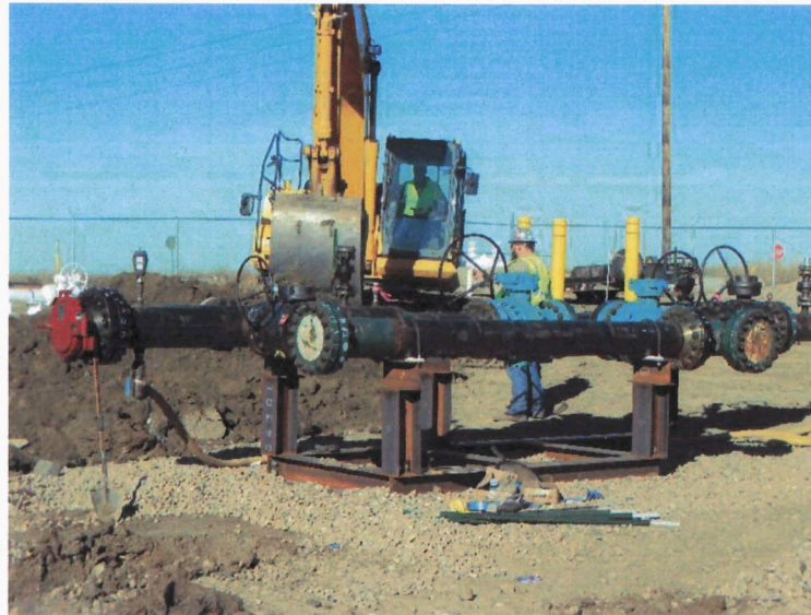
Picture 3 – Preparation for final tie-in of Global Stampede Pipeline to Divide Lateral Pipeline near Fortuna, ND
