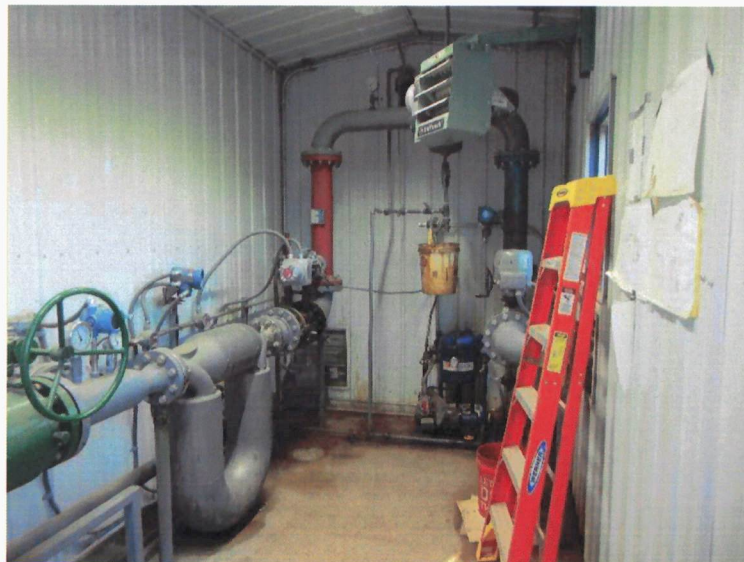
Picture 2 – General Piping Layout inside LACT near Epping, ND
