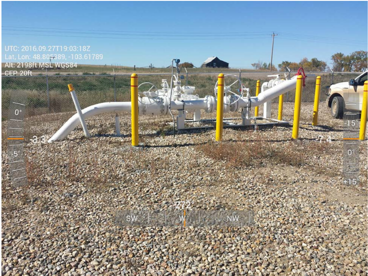
Photo 11 – End valve, connecting to Divide Pump Station.
