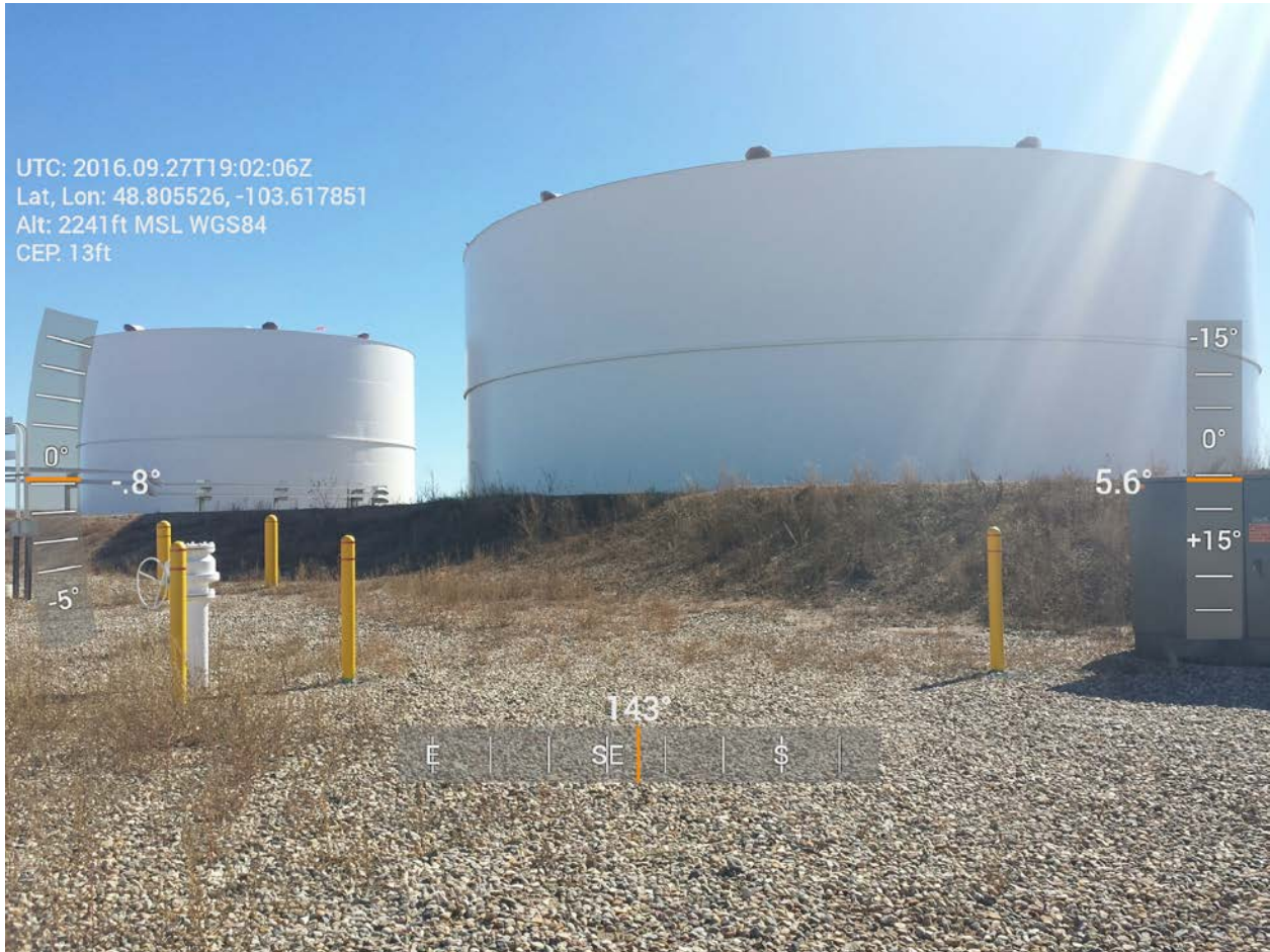
Photo 10 – Tanks at the Divide Pump Station.
