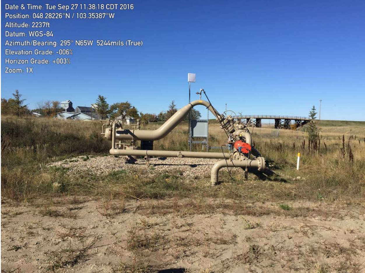
Photo 1 – “PIG” launcher at CRT, pipeline start.
