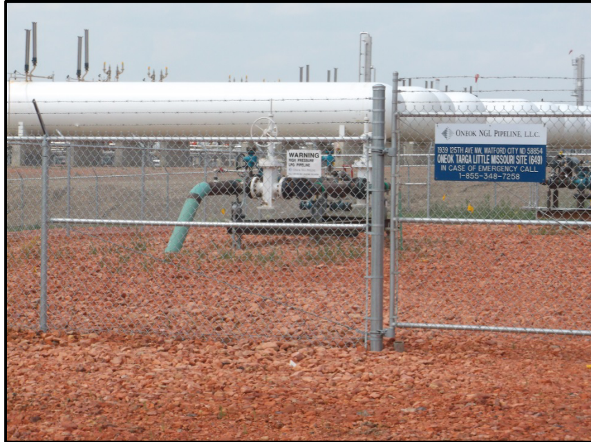
Photo 1. Direction: Northwest. Pipeline with pig launcher, leaving the ONEOK Targa Little Missouri Site.
