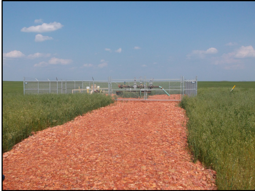
Photo 25. Direction: East. Pictured above is the pig receiver and the end of the Targa Lateral Pipeline Project.
