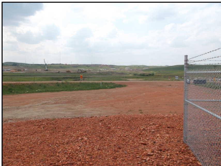
Photo 2. Direction: West. Row and pipeline corridor running east to west approaching the first crossing of an access road.
