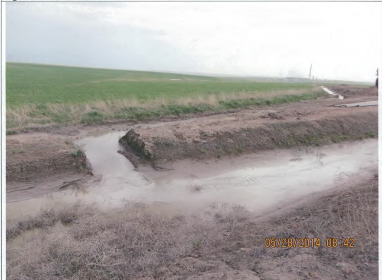
Figure 2: Washed out berm
