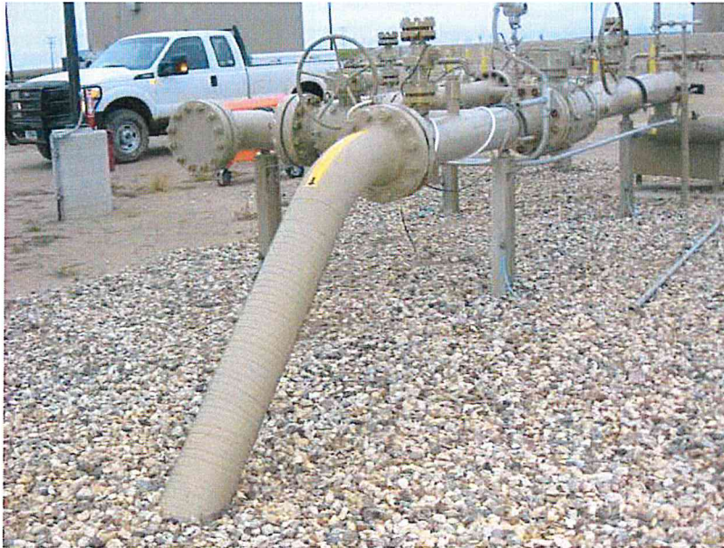
Photo 4 – View of 8" pipeline interconnect at New Town tank facilities.
