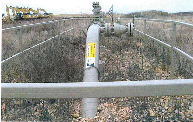
Photo 11 – Approx. Station 1230+00. View of Mainline Block Valve.
