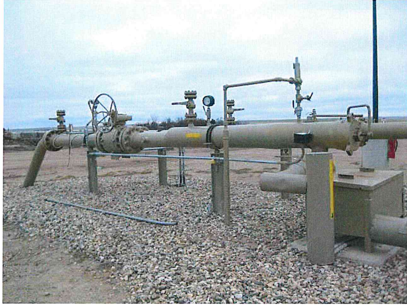
Photo 3 – View of 8" pipeline interconnect at New Town tank facilities.
