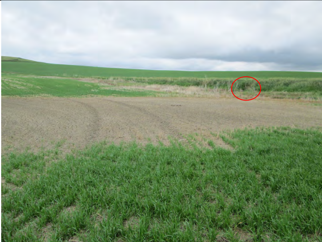
Photo Point 7 – Area of sparse vegetation and surface cracks indicating surface ponding. Culvert under road indicated by circle.
