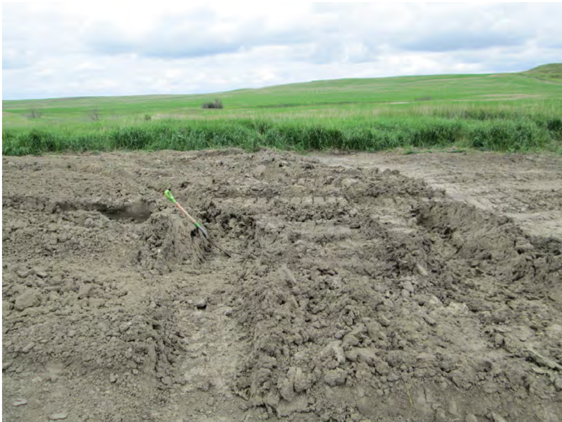
Photo Point 10 – Pipeline crossing location of Wetland 02, note severe rutting indicating saturated soil conditions
