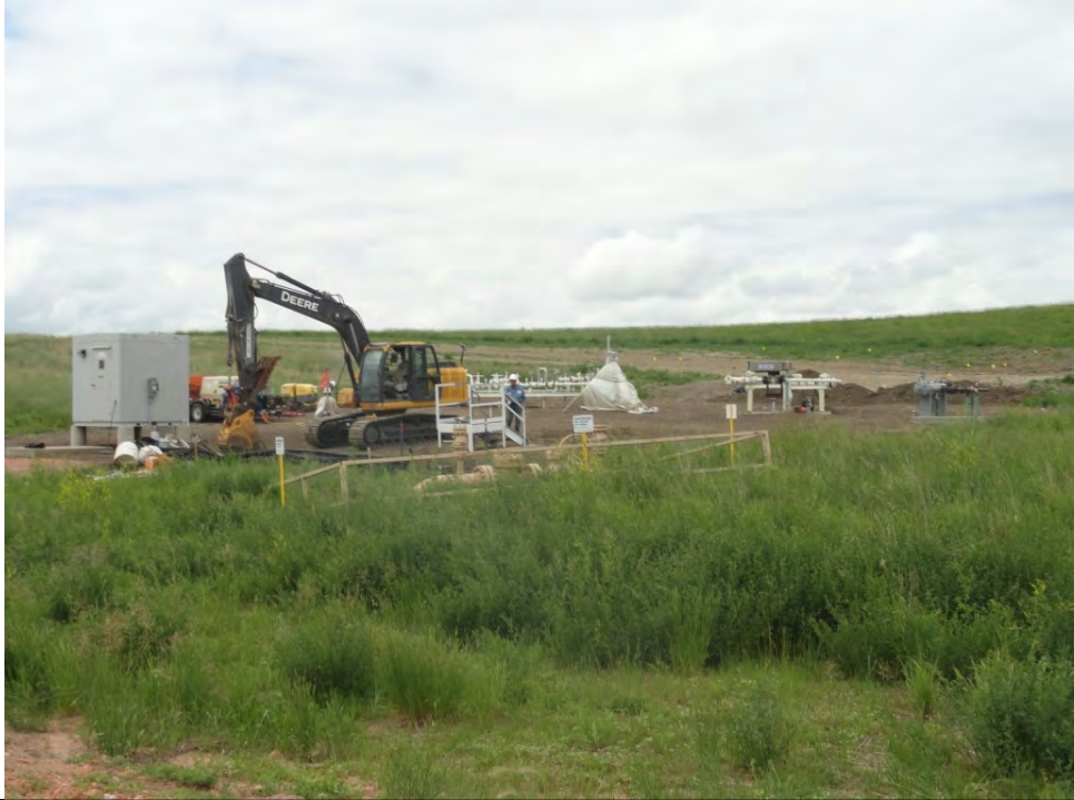
Photo Log Point 14: Pipeline terminus OneOK
