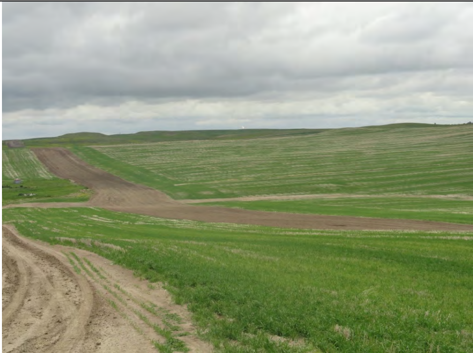
Photo Log Point 9: Pipeline route looking north (Hey Butte facility flare in background)
