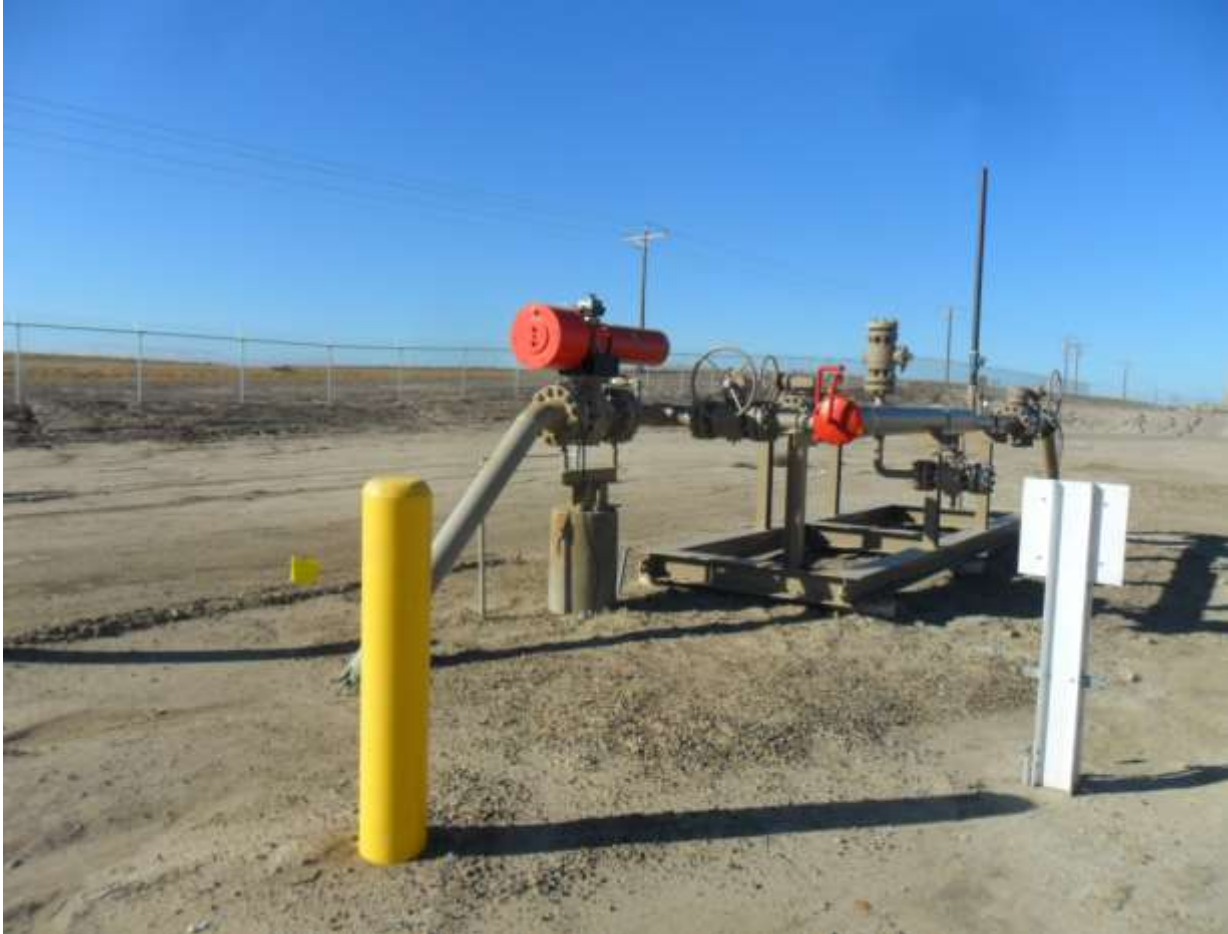
Photo 1 – “PIG” launcher at Hay Butte Plant, pipeline start.
