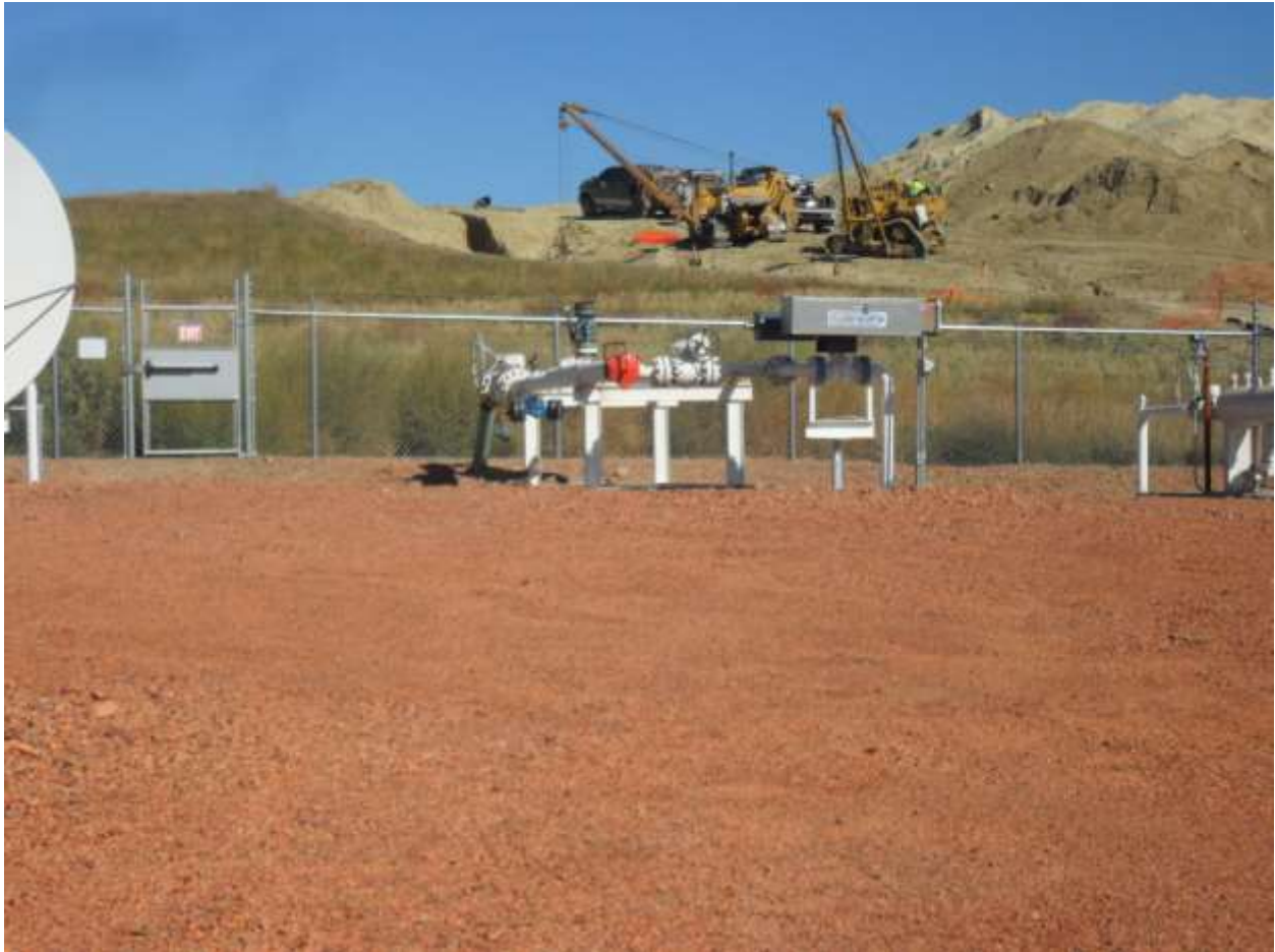
Photo 11 – End valve, connecting to ONEOK Partners’ Bakken NGL pipeline.
