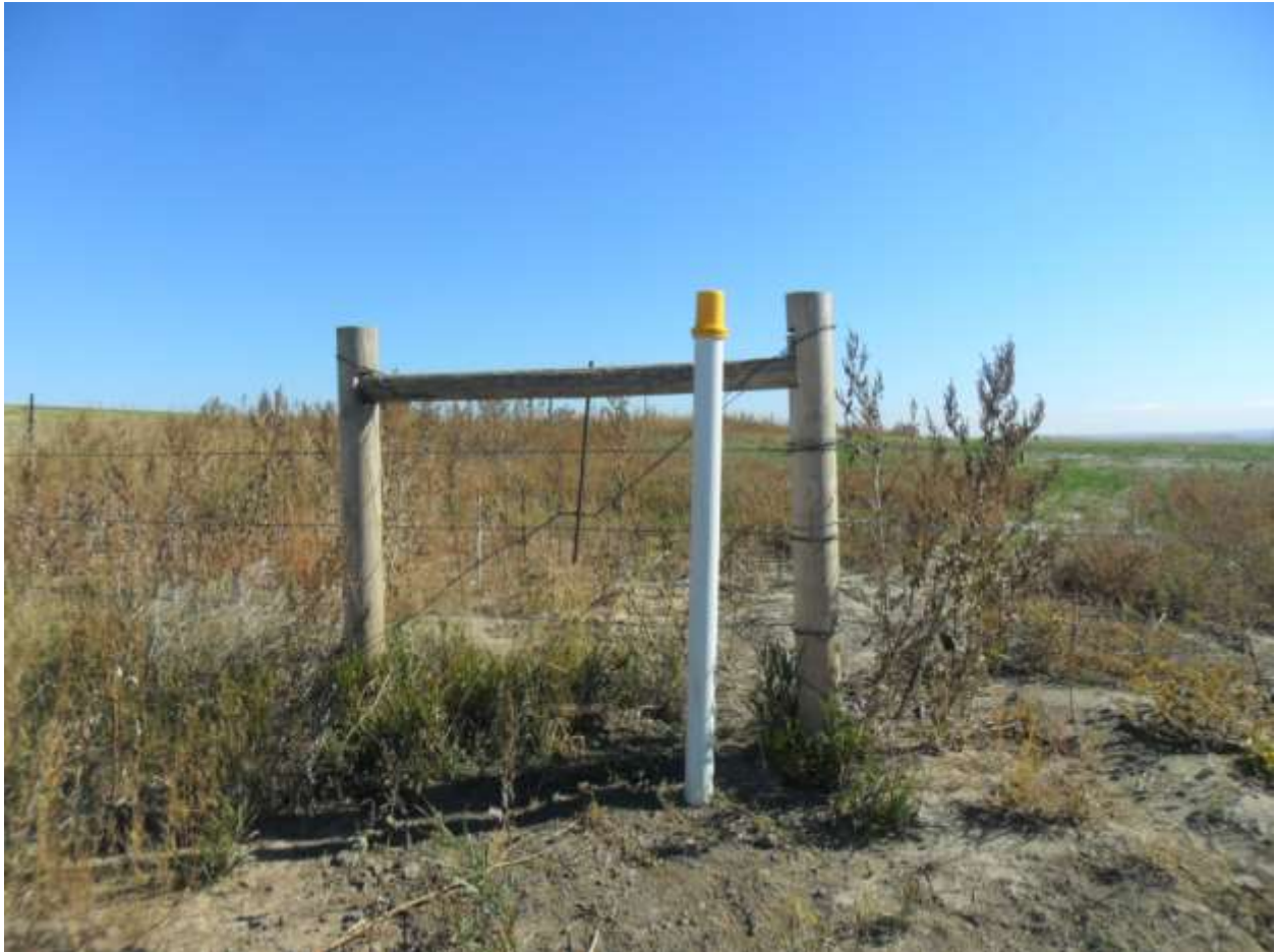
Photo 6 – Pipeline marker at fence crossing.
