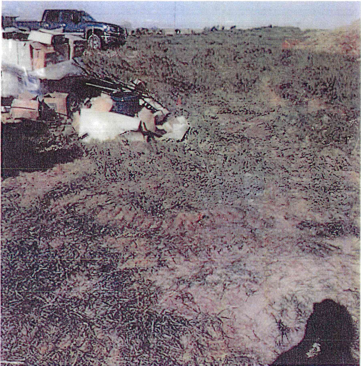
Standing on location of damage looking north, the flags are marking the fiber line that was located west of the line that was damaged
