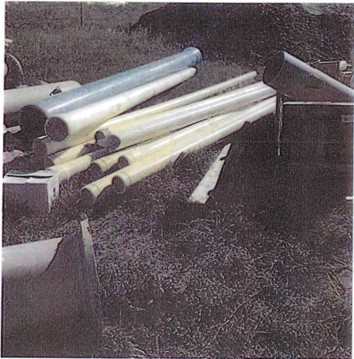
Old flag found under pipe marking fiber that was hit, flags were from previous locate by Carstensen Construction on May 13, 2014 to install the Booster Station Ticket 14057188, our locates was submitted 07/01/2014 Ticket 14094811. This was 54 feet north of the damage. These flags were not visible from the location of the Directional Drill
