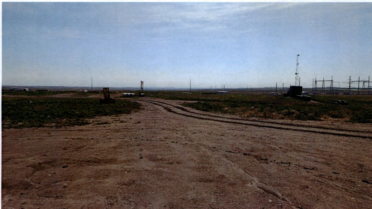
Photo 1. Substation on west end of Project, with stored equipment in the background.
