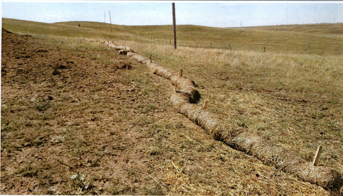
Photo 3. Properly-installed waddle on downhill slope of crane pad.
