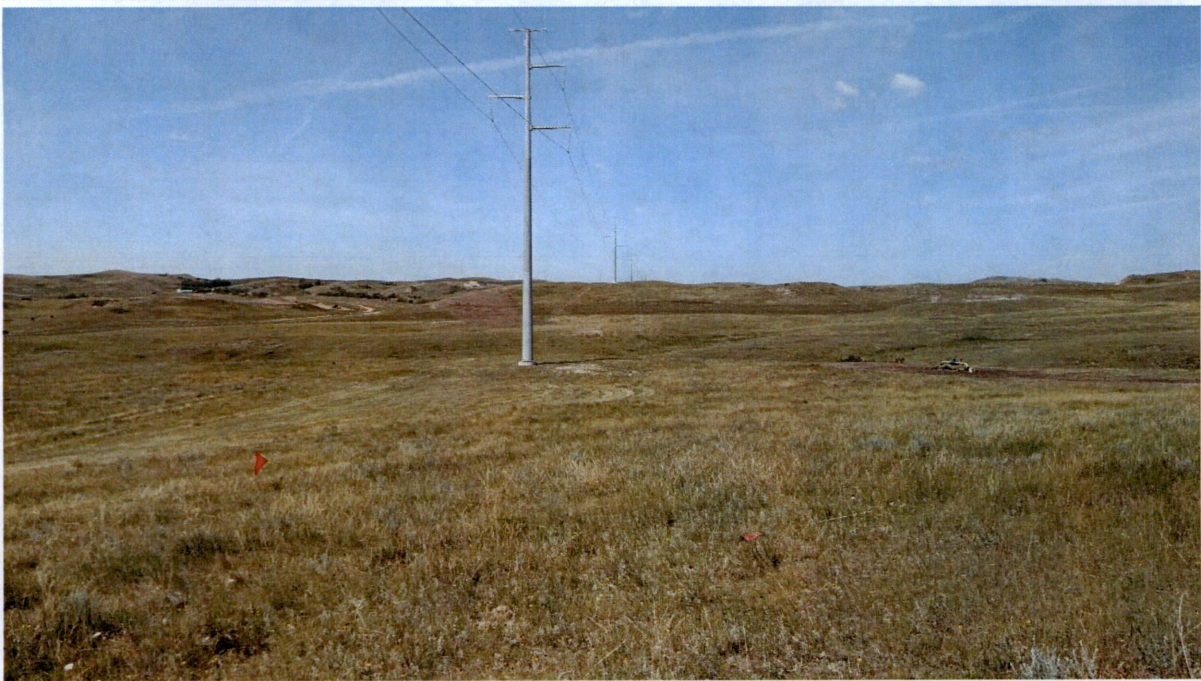
Photo 5. Strung towers spanning recent pipeline project.
