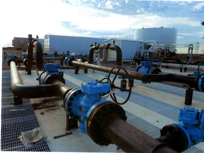
Picture 2 - Piping serving future truck LACT area
