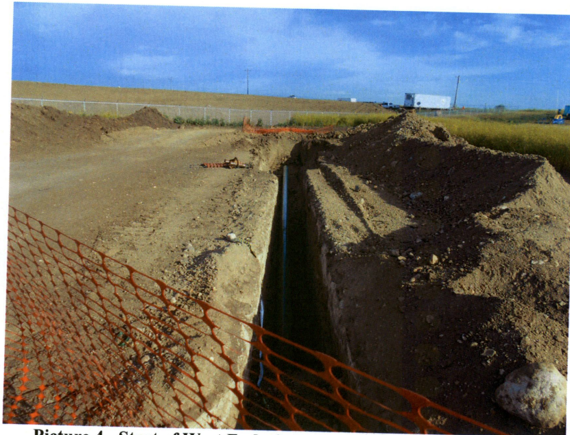
Picture 4 - Start of West End of pipeline. Notice soil segregation.
