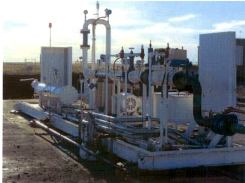
Picture 2 - Piping serving future truck LACT area
