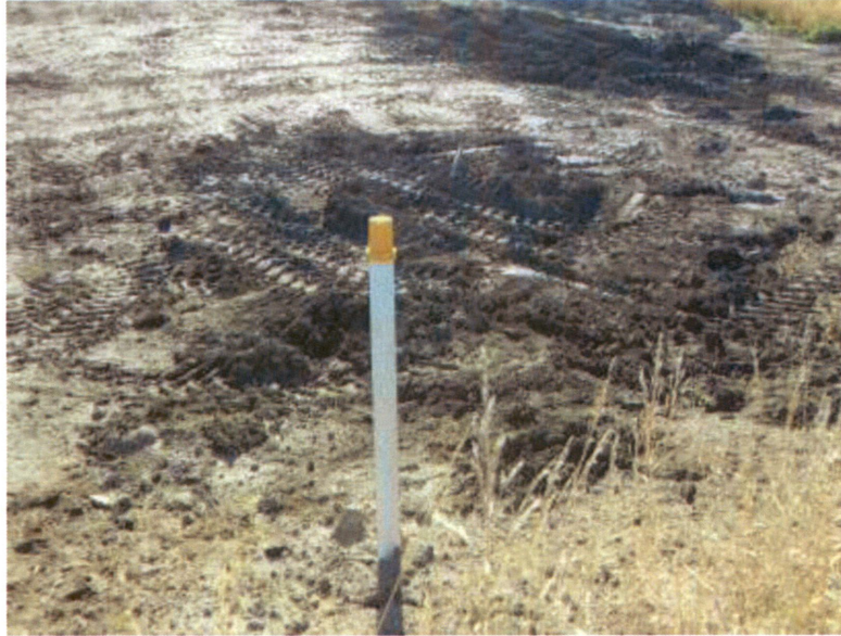
Picture 5 - Typical piping cathodic protection point
