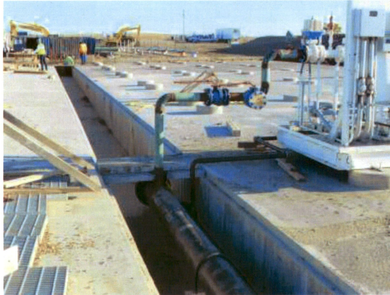
Picture 3 - Tractor Trailer LACT area west end of pipeline
