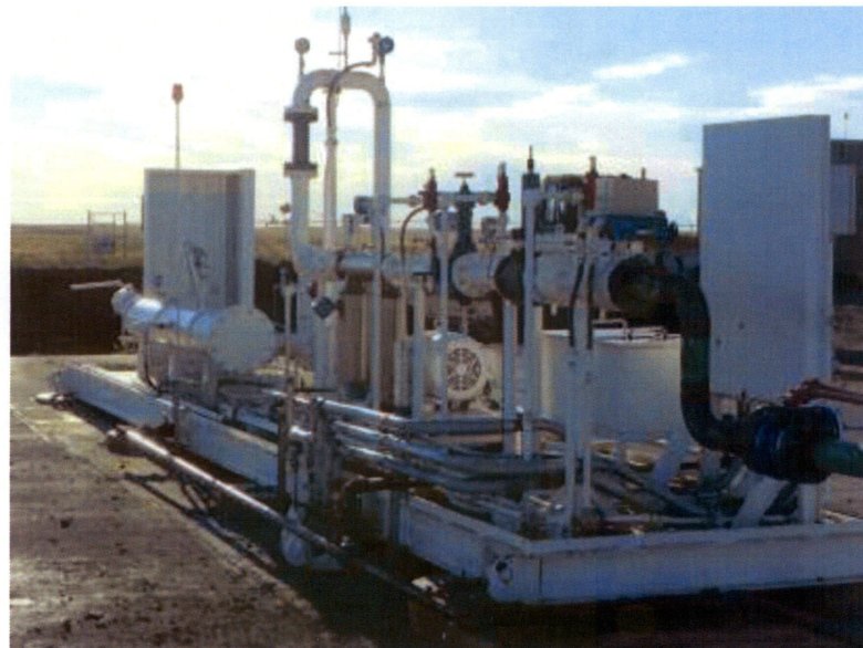
Picture 2 - Piping serving future truck LACT area
