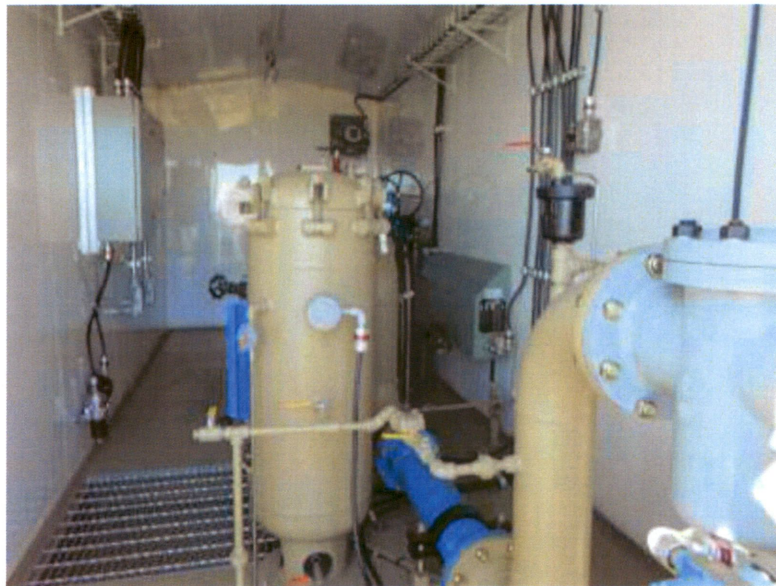
Picture 10 - Inside view of LACT on east side of pipeline
