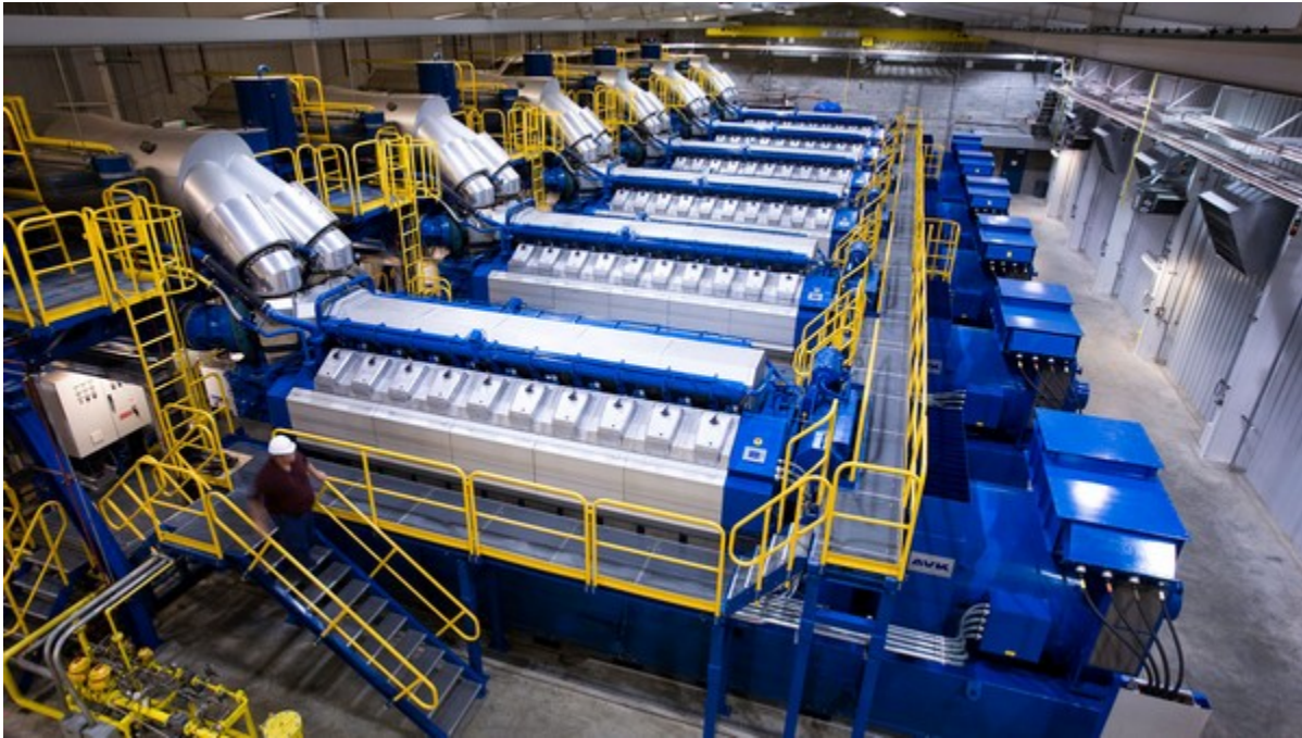
Figure 1-18: Engine Hall at Goodman Energy Center in Kansas
