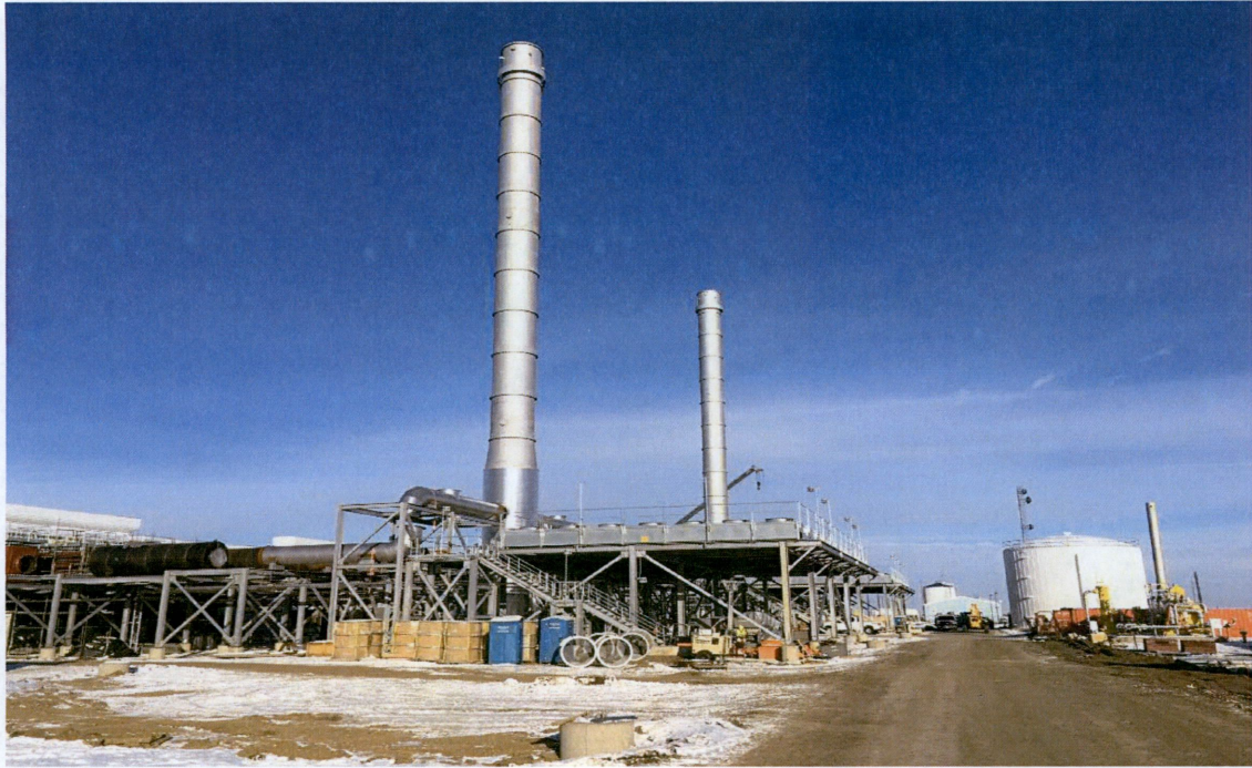
Photo 1 – View of Pioneer Generation Station Phase III facilities
