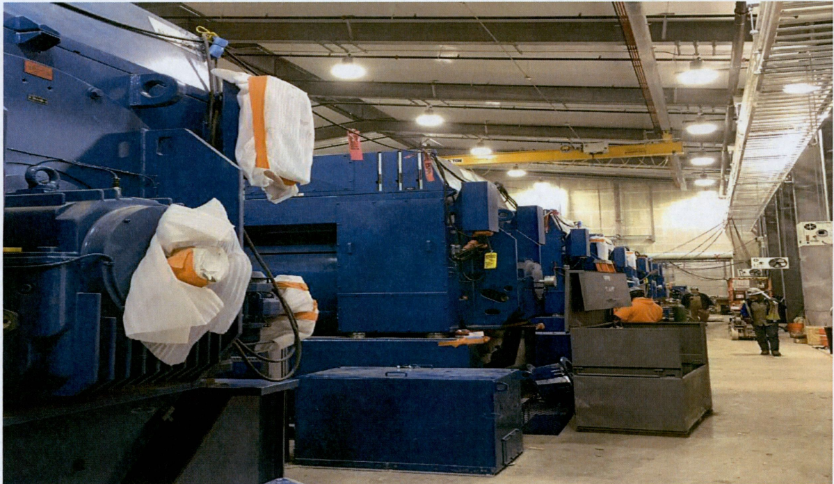
Photo 4 – View of engines in the South Engine Building
