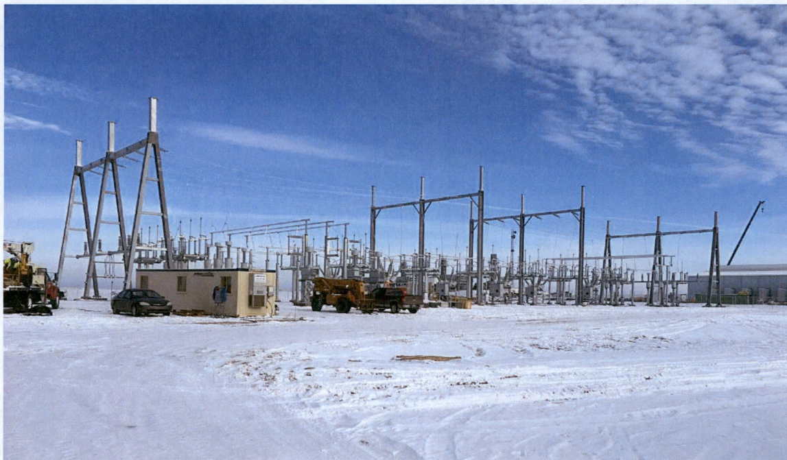
Photo 10 – View of switchyard
