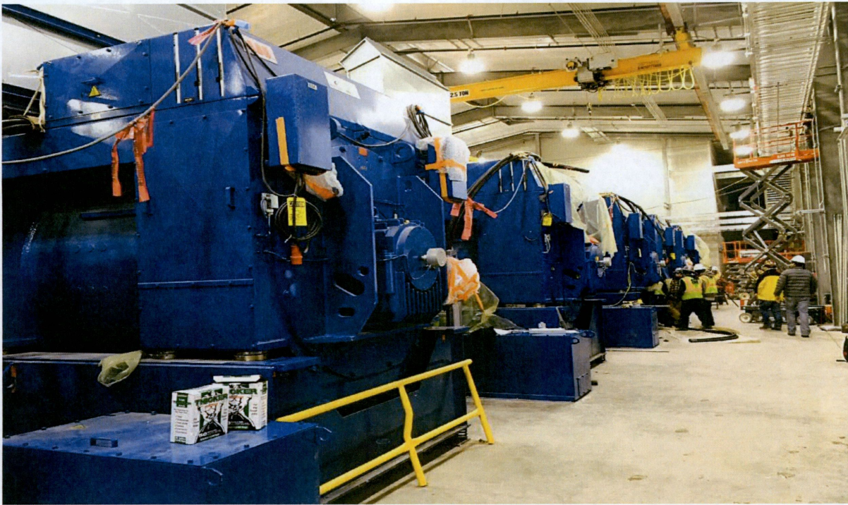
Photo 3 – View of engines in the North Engine Building
