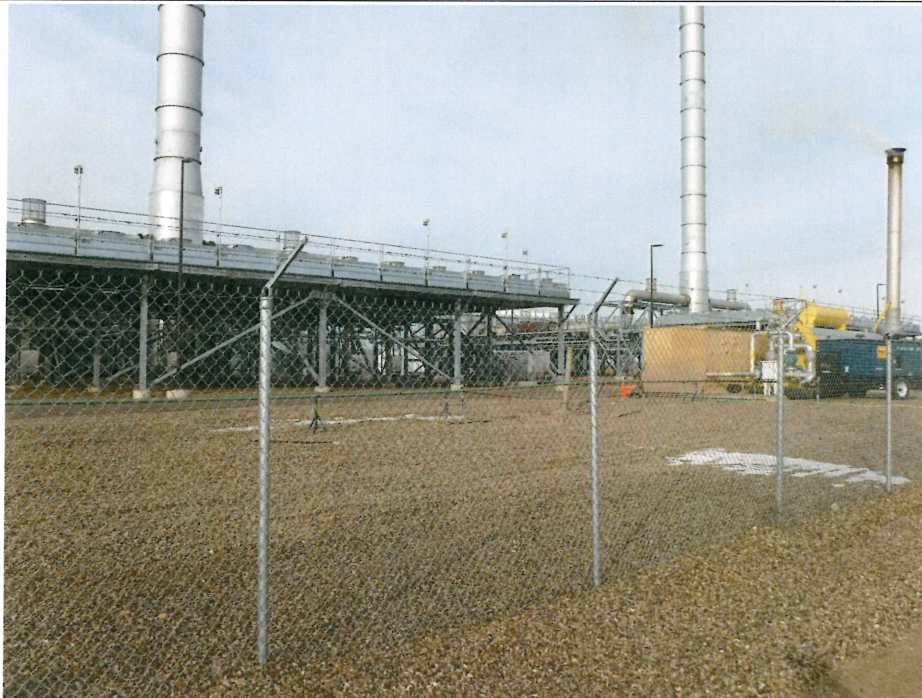
Photo 4 – View of Pioneer Generation Station Phase III facilities.
