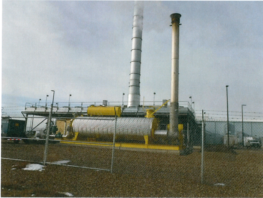
Photo 3 – View of Pioneer Generation Station Phase III facilities.
