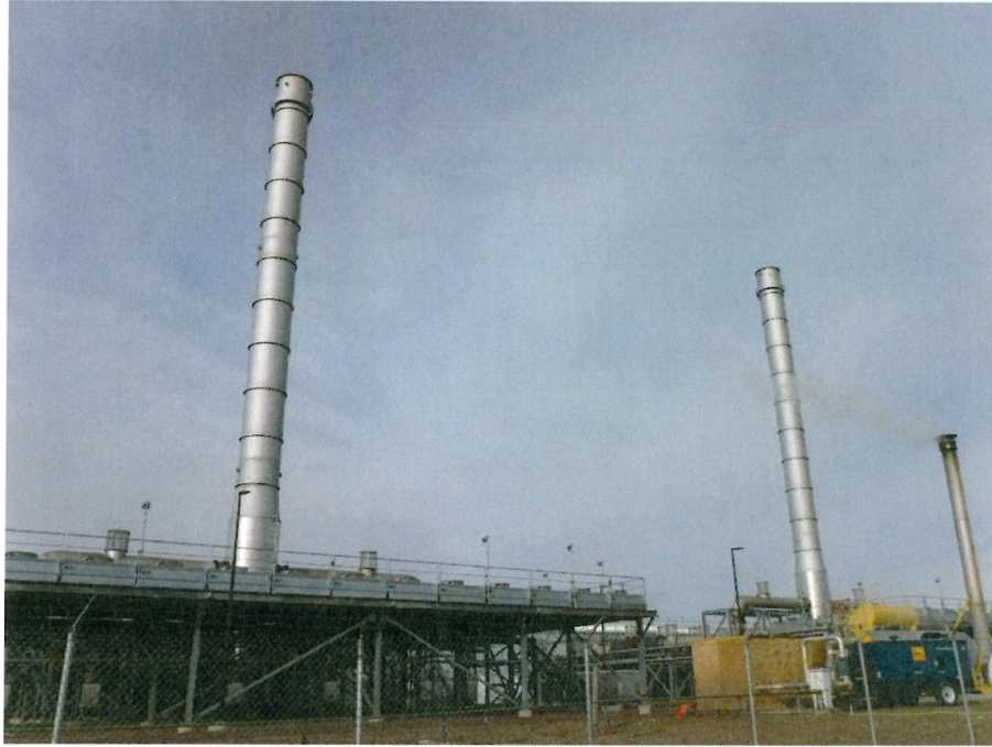
Photo 1 – View of Pioneer Generation Station Phase III facilities.
