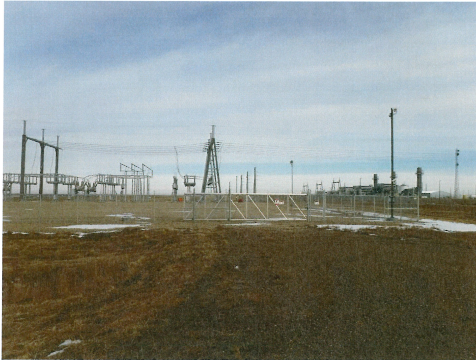
Photo 5 – View of switchyard.
