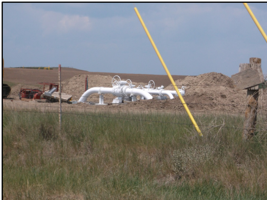
Photo 22. Direction: Southwest. After crossing 36 th St NW the pipeline bends back to the east and runs parallel to the road on the south side. Pictured above is another active construction site at a block valve at the time of the inspection.
