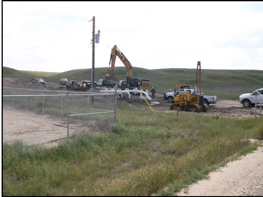
Photo 25. Direction: South. This is a third active construction site at the time of the inspection. It is likely that construction has been completed since the inspection and it is recommended that the PSC follow up with Kinder Morgan.
