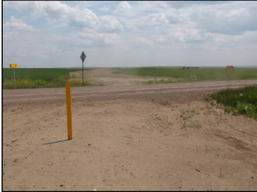
Photo 29. Direction: East. This is the section of the pipeline corridor that runs east and west parallel to 36 th St NW. The ROW along the road has not been completely reclaimed. Shown here is an access road crossing that was completed by boring underneath the road. Also shown is an above ground pipeline marker.
