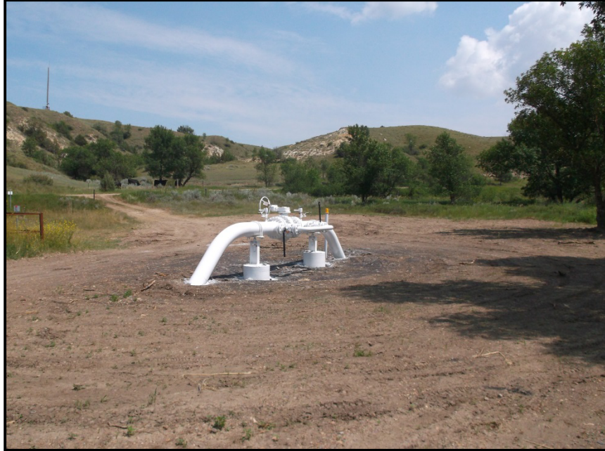
Photo 15. Direction: Northeast. Pictured above is one of several block valves, at this point the pipeline bends to the north. This area also still needs to be seeded.
