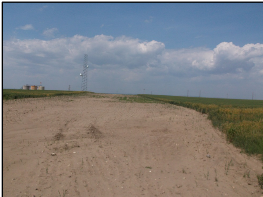
Photo 28. Direction: East. This portion of the corridor was recently seeded and needs to be monitored until fully reclaimed. It was apparent that the route corridor widths described in the application were used throughout the project as depicted in the picture above.
