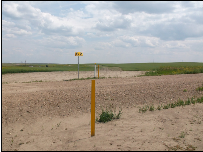
Photo 31. Direction: East. This is the section of the pipeline corridor that runs east and west parallel to 36 th St NW. The ROW along the road has not been completely reclaimed. Shown here is an access road crossing that was completed by boring underneath the road. Also shown are above ground pipeline markers.
