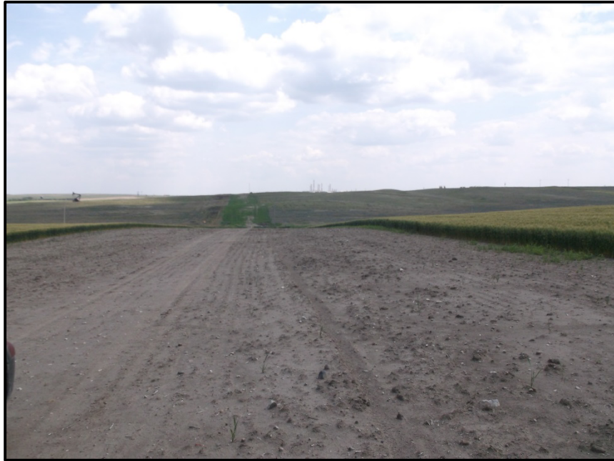
Photo 33. Direction: East. Another section of the pipeline corridor running east and west that has been recently seeded and should continue to be monitored until fully reclaimed.
