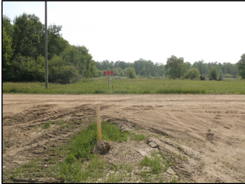
Photo 9. Direction: East. This is the entry point for the bore underneath the Yellowstone River.
