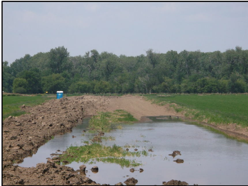
Photo 10. Direction: West. This is the exit point for the bore underneath the Yellowstone River. At the time of the inspection the topsoil was being put back in place. Standing water is a result of irrigation from surrounding farmlands. Area will be completely mitigated by the end of construction.
