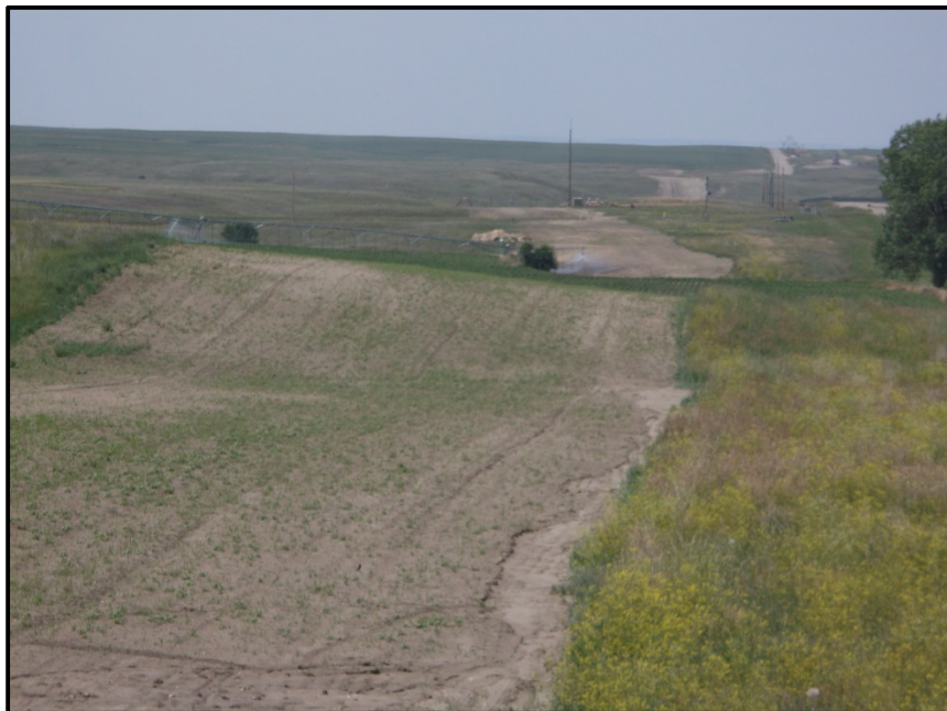
Photo 26. Direction: East. This portion of the corridor was recently seeded and needs to be monitored until fully reclaimed. It was apparent that the route corridor widths described in the application were used throughout the project as depicted in the picture above.
