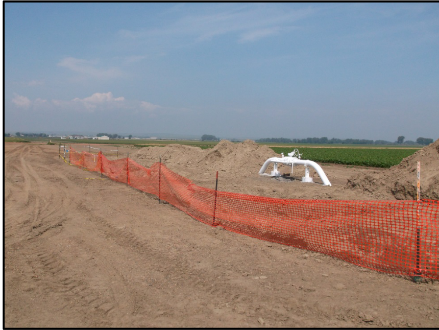
Photo 7. Direction: Northwest. One of several currently active construction sites that will be completed in the near future. Pipeline continues to run east along the ROW.
