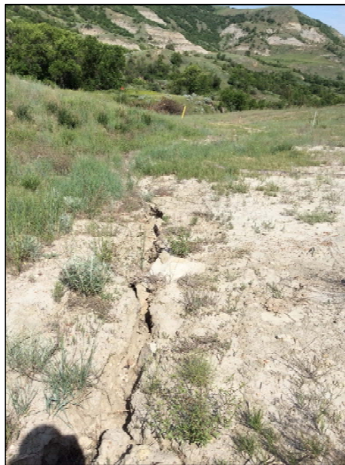
Photograph 8. Incising stream channel across eastern edge of ROW fill. View to northwest.
