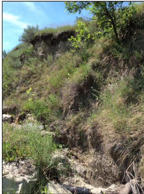
Photograph 12. 12-foot-tall embankment along western margin of fill area. CMP drainpipe at bottom of photo. View to south.
