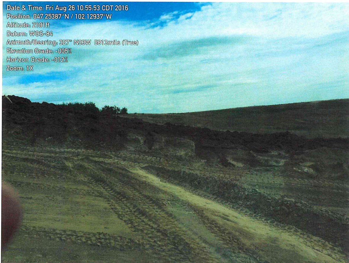
Photo 3 -Subsoil cast on topsoil likely during flow-breaker install at 47.2539°N -102.1294°W.
