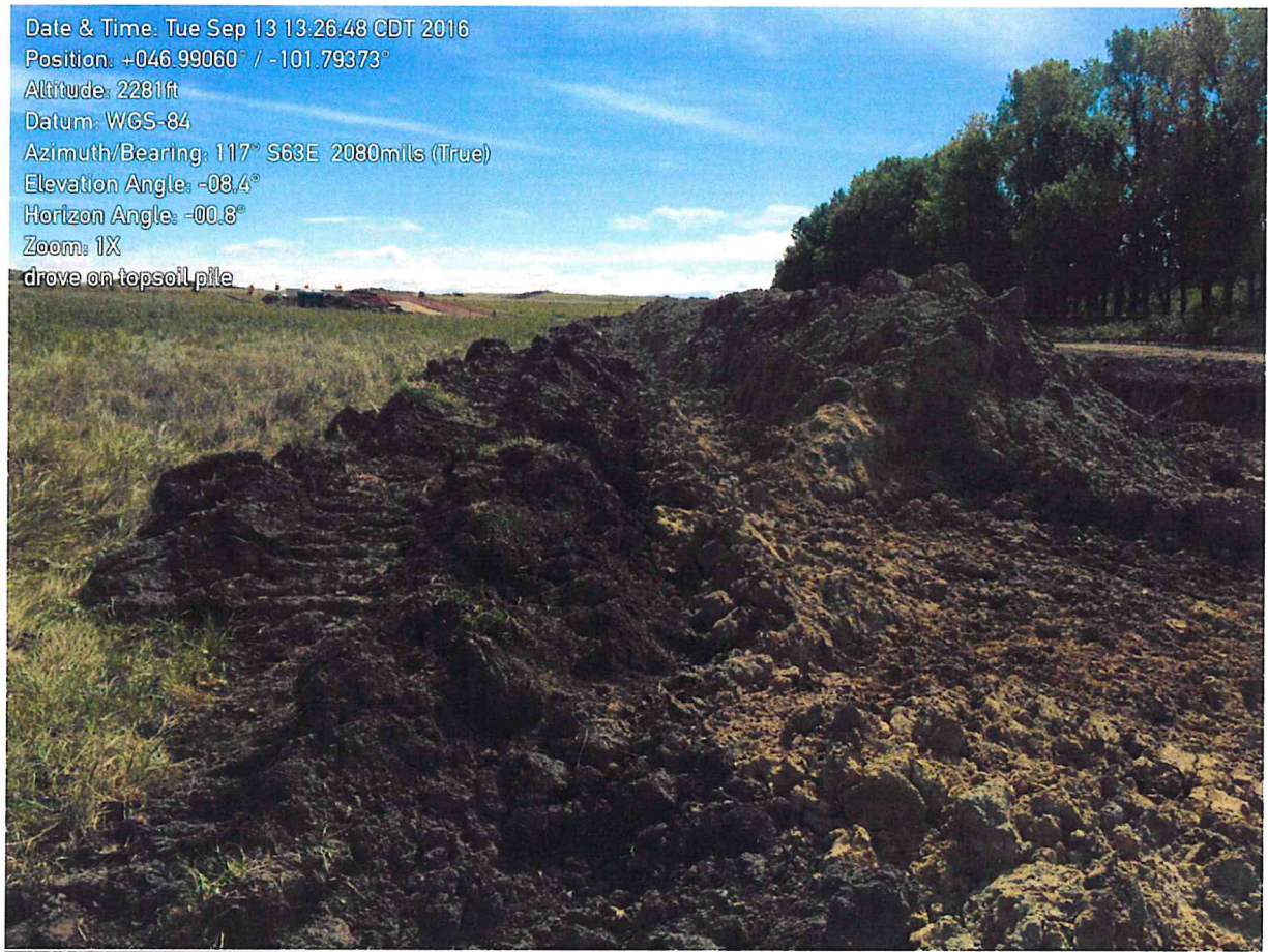
Photo 4 -Topsoil and subsoil piles mixed by equipment traffic at 46.99060°N -101.79373°W.
