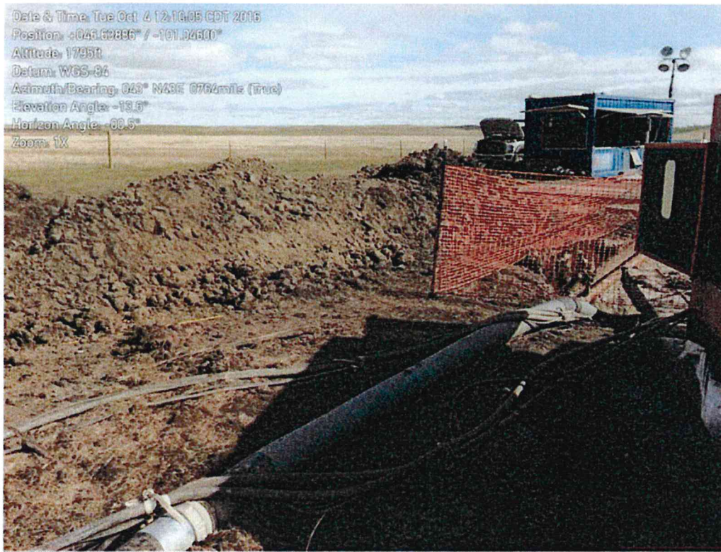
Report Photo #2 "Subsoils from HDD Bore Entry Pit on Unstripped Ground: 46.63866°N 101.04600°W
